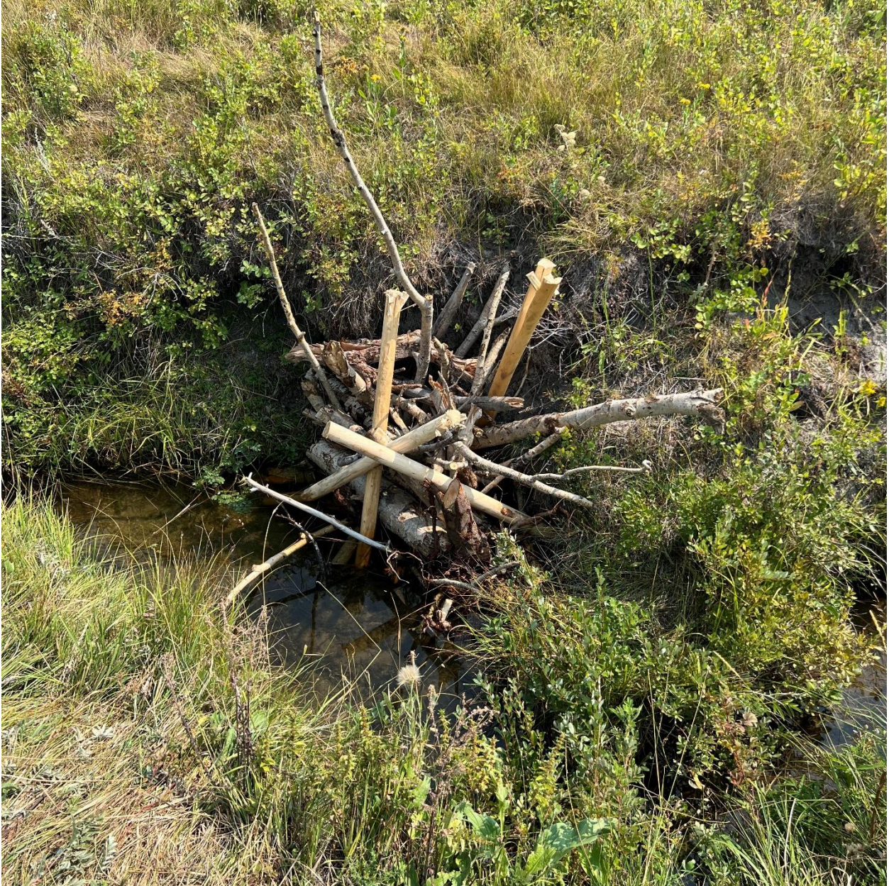
Figure 6. This Low-Tech Process Based restoration structure recently installed by SRWG on Arnold Coulee will reduce sediment from entering the stream while the bank builds back up and vegetation fills back in. Similar strategies are suggested for the Muddy Creek basin.
