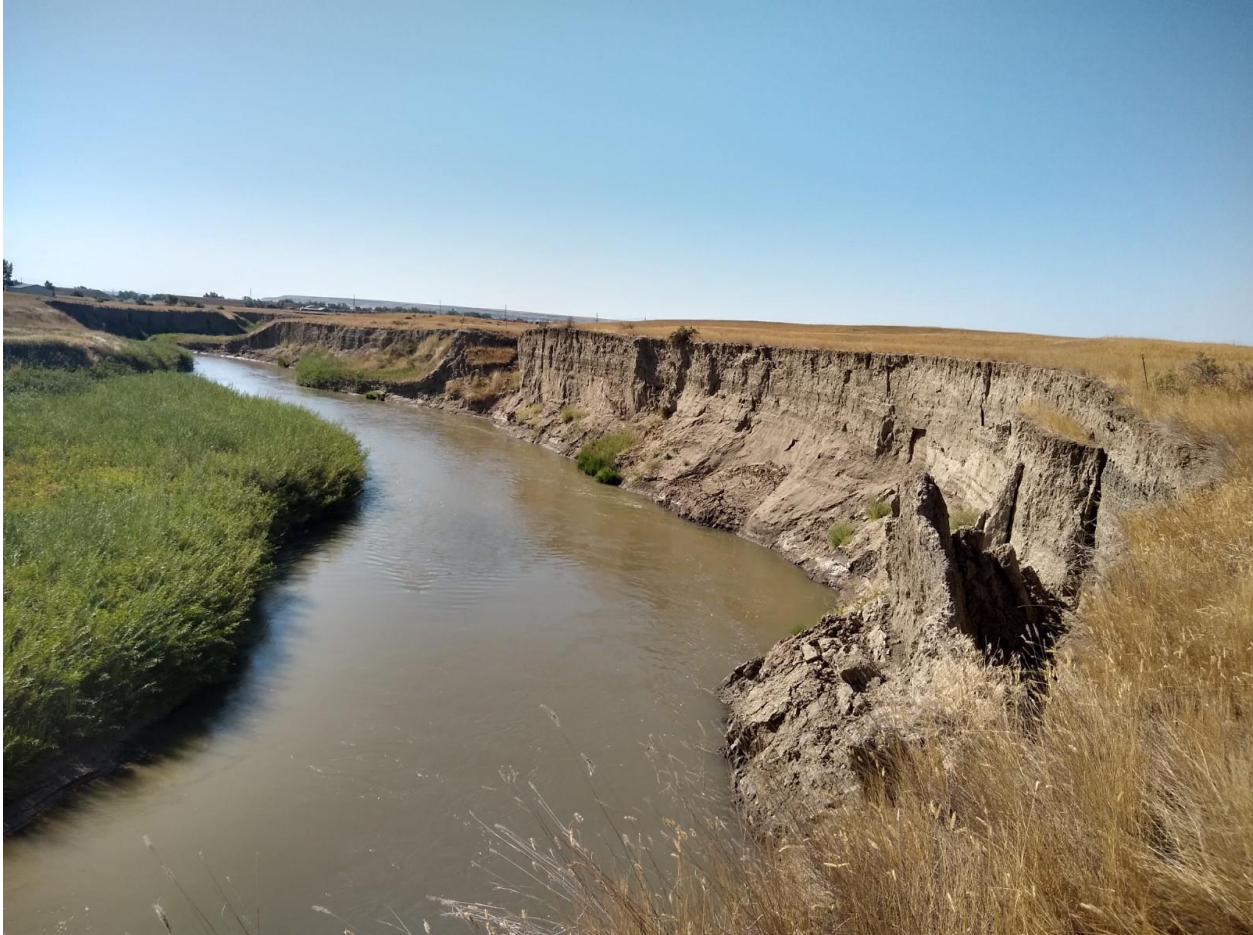
Figure 5. Muddy Creek. To the right, dry vegetation and collapsing banks (contributing to poor water quality) are characteristic of an incised channel and disconnected floodplain. On the left where floodplain is connected, vegetation is healthy and banks are stable.
