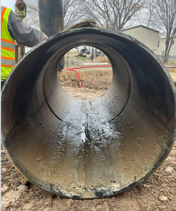
Inside of pipe section removed where new access way will be installed in preparation for cleaning and inspection.
