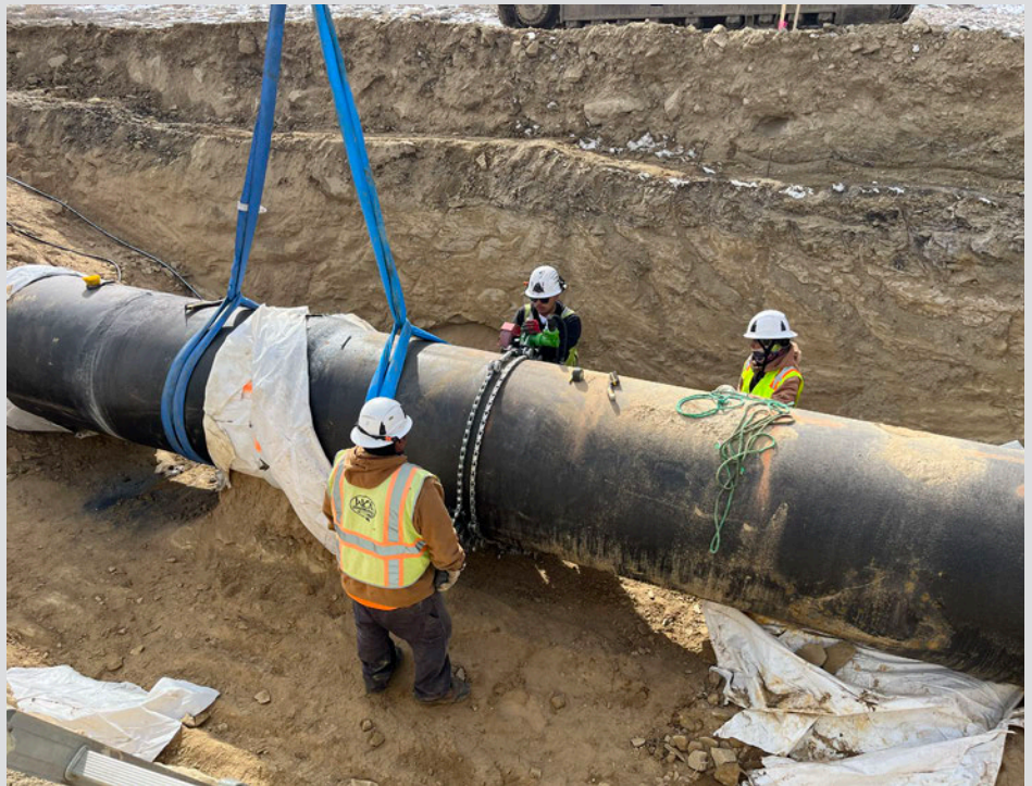
WCA crew preparing to remove section of pipe at location of plunger valve to prepare for cleaning and inspection.
