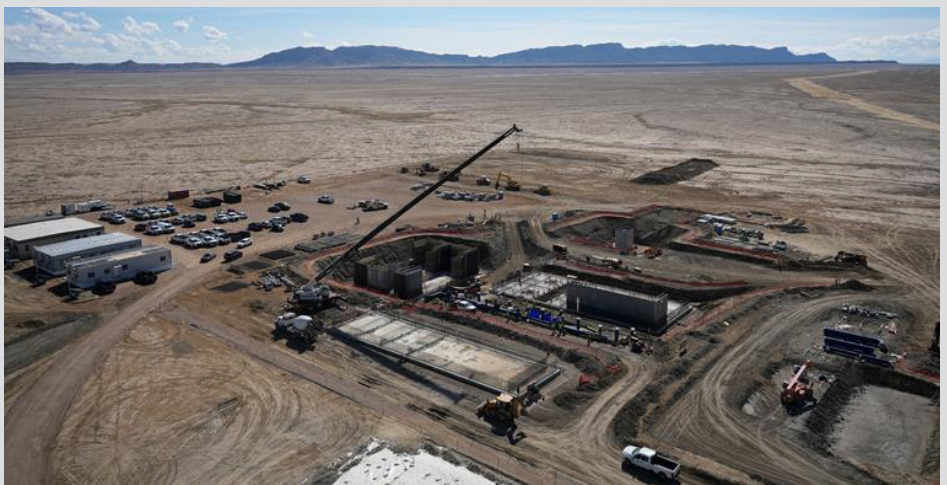
Aerial photo of active construction at the water treatment plant located off HWY N-36.
