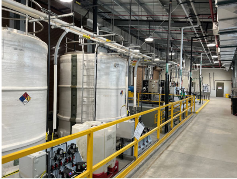
Cutter Lateral Water Treatment Plant – Coagulant storage tanks within the chemical building.
