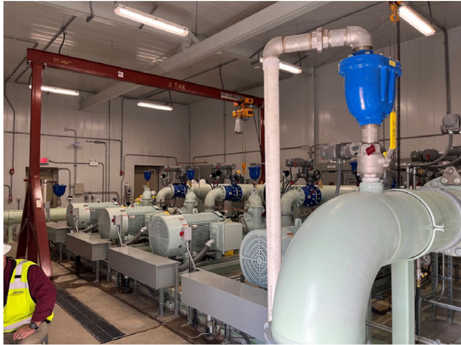
Cutter Lateral – Interior of a raw water system pumping plant.
