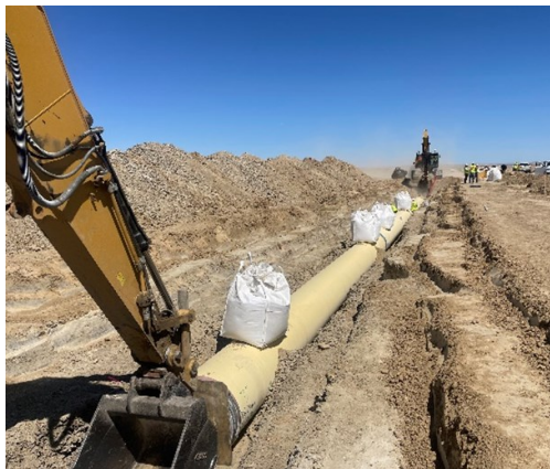
NGWSP - Block 4A/B – Installation of the 42-inch steel pipe. After the pipe is in the ground, contractor will backfill 2/3 of the pipe with a material that is a mixture of soils with cement (Its call Controlled Low Strength Material (CLSM)). The sandbags are used to prevent the pipe from floating during CLSM placement. Photo by Hilda Castillo Smith
