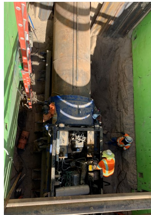
Code Talkers Sublateral (Reaches 12.1/12.2) – Photo shows the auger boring machine setup at the launching shaft or entry pit. This auger boring was for a 48-inch casing pipe. Photo by Hilda Castillo Smith
