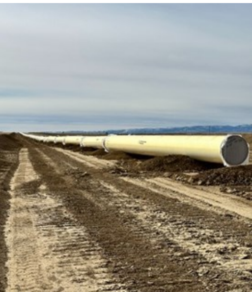
NGWSP - Block 4A/B – Once the 42-inch steel pipe gets delivered to the job site, the contractor will string the pipe along the construction ROW. Photo by Hilda Castillo Smith.
