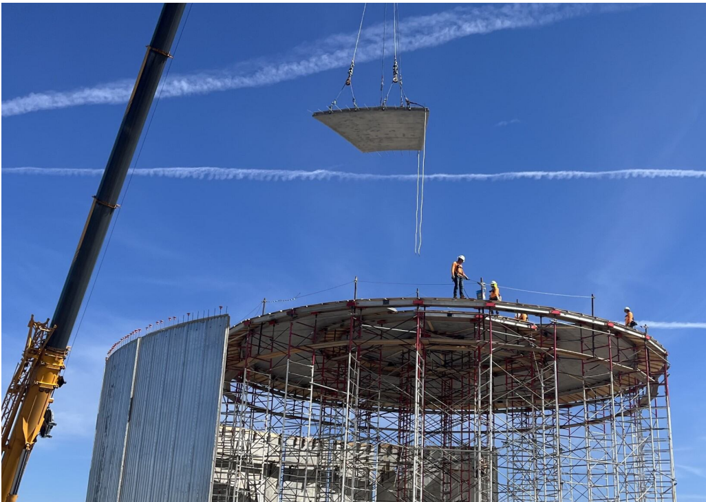
NGWSP- Reach 12.1 SJ Louis subcontractor DN Tanks installs the roof dome panes to Black Hat Tank. Photo by Vicki Cassidy on 6/28/2024.
