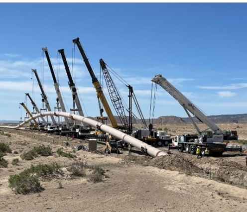
NGWSP - Block 4c - 8 – Crossing of a large wash using Horizontal Directional Drilling. The picture shows eight (8) cranes lifting the 48-inch steel pipe before it gets pulled from the other side of the wash. Photo by Hilda Castillo Smith.
