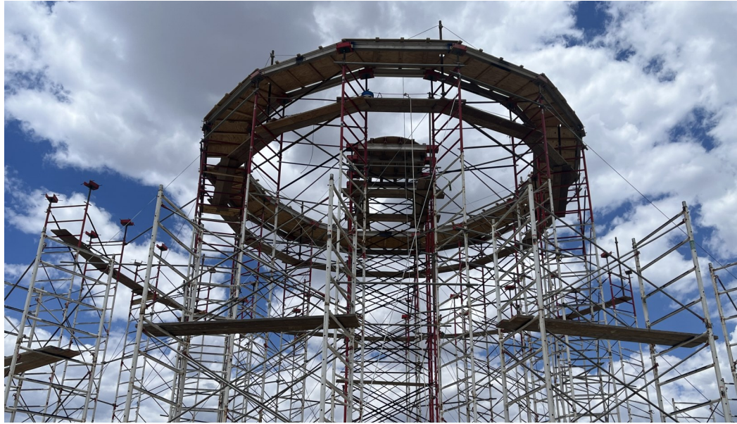
The scaffolding and shoring being installed at Black Hat Tank. They will be used to install the wall and dome panels that are cast on site with concrete. Photos by Paul Bergstrom.
