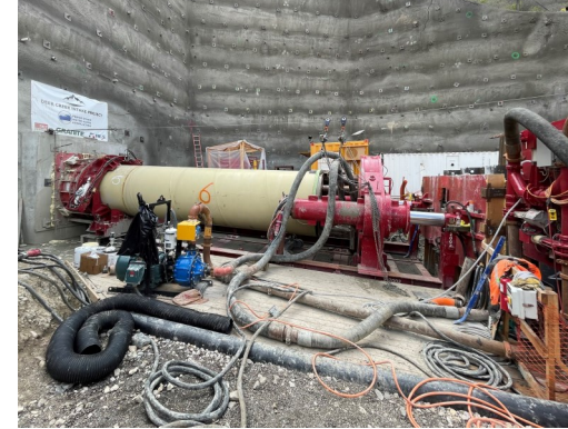
An example of a microtunnel boring machine (MTBM) entry portal. This equipment is currently being used on Reclamation's Deer Creek Intake Project, in Utah. The MTBM excavates the tunnel while simultaneously installing the pipeline. Guided by a laser and using a slurry to carry away excavated material and keep the tunnel face stable, the machine moves about 20 feet or one pipe section per day. Reclamation photo
