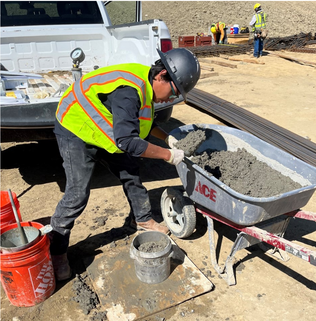
FCCO Lab Technician Isaiah Smith tests concrete for specification compliance. Reclamation photo by Brad Gordanier
