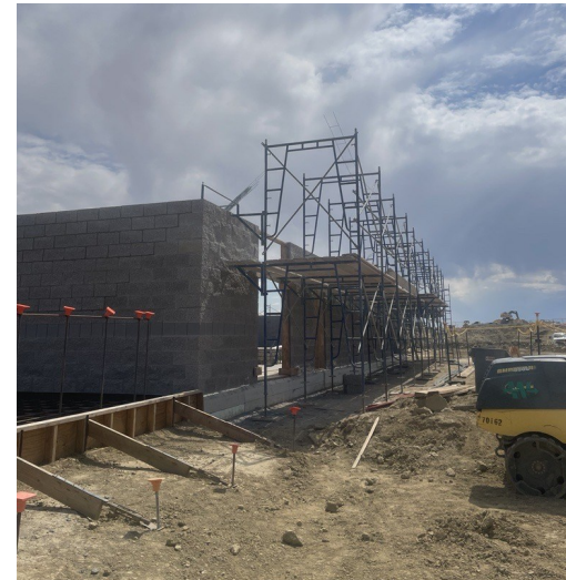
Concrete blocks being installed to form exterior walls at Pumping Plant 3. Reclamation Photo by Hilda Castillo Smith
