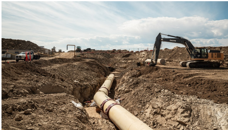
Construction underway on the Navajo-Gallup Water Supply Project in the Santostee Chapter, south of Shiprock. Reclamation photo by Pablo Mena
