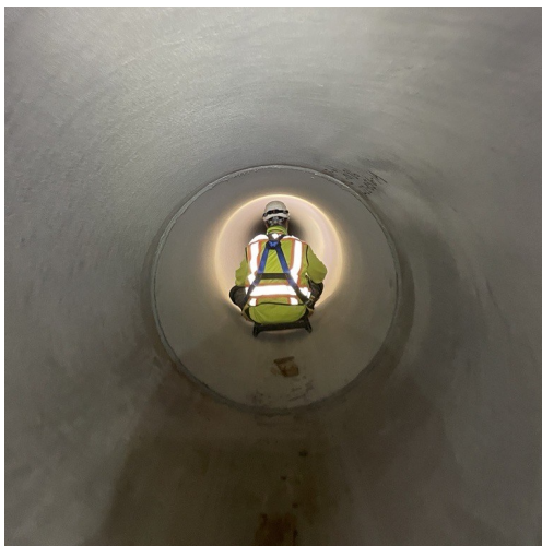
HB- Four Corners Construction Office employee Bradley inspects inside of pipe on Reach 4B. Reclamation Photo by Hilda Castillo Smith
