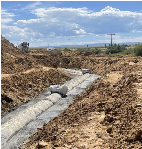
HB- A 42-inch pipeline being installed at Reach 4B. Reclamation Photo by Hilda Castillo Smith
