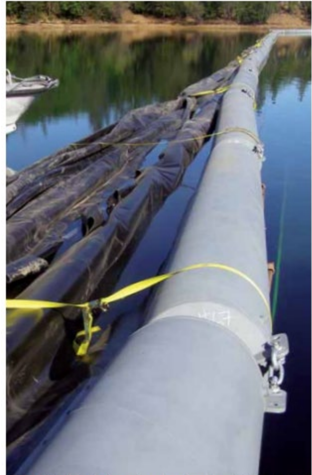
FIGURE 8 Metal floats in place and curtain ready to be anchored to the river bottom by 800-lb weights
