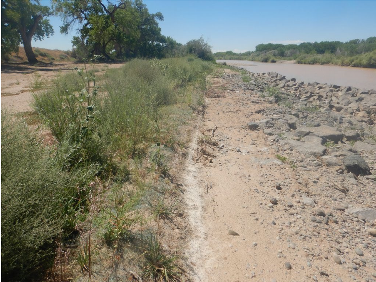
Figure 7: Looking downstream from same vantage point as in previous figure at the longitudinal stone toe protection on the eastern bankline; photo taken post-runoff 2023 (Wolf Engineering, 2023)
