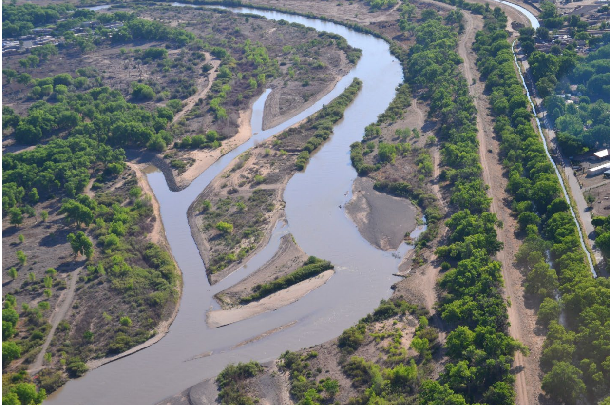
Figure 8: Construction of new side channels on the western floodplain of the Sandia Priority Site (Reclamation, 2023)
