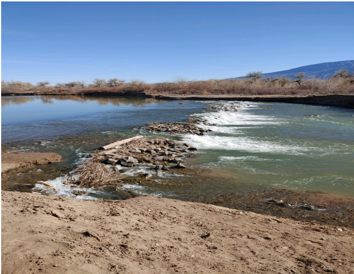
Figure 10: Looking east at the Corrales Siphon and the 2020 riprap protection placed downstream of the siphon (Reclamation, 2023)
