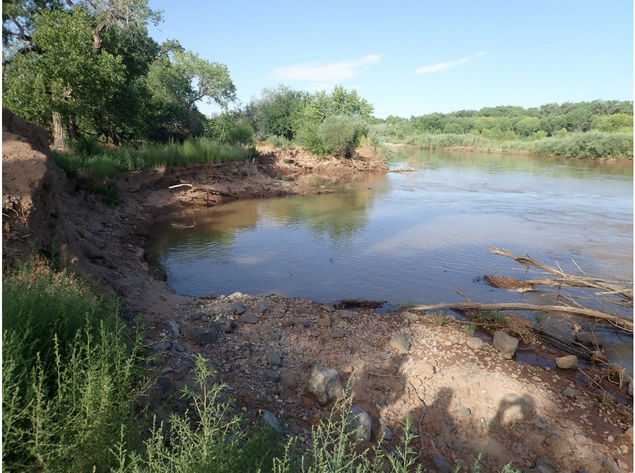
Figure 6: Looking downstream at Santa Ana RM 205.8 east bankline bendway weirs prior to 2023 repairs (Reclamation, 2021)
