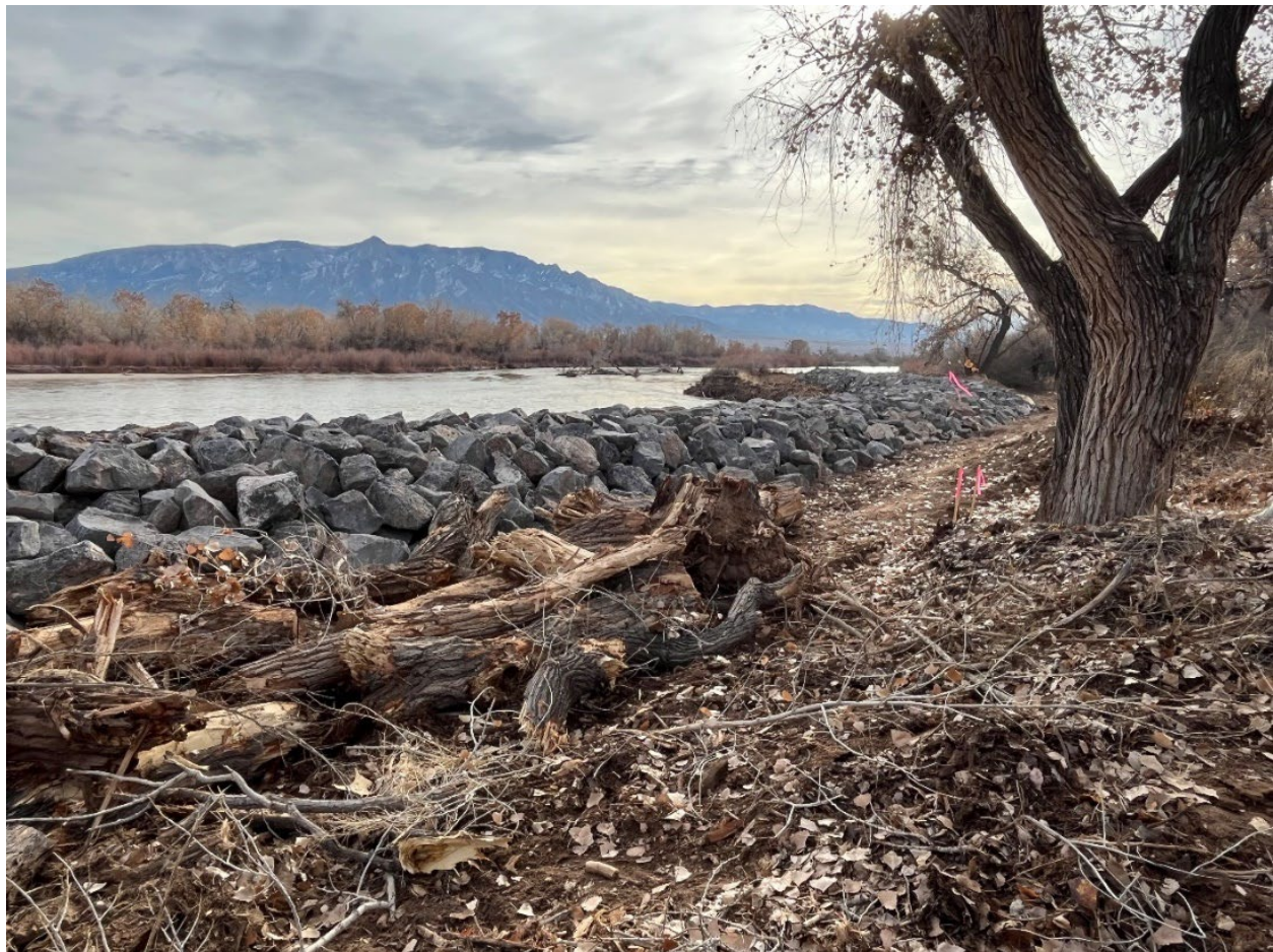
Figure 13: Riprap windrow constructed along the eroded bankline at the Corrales Siphon Bend (Reclamation, 2024).
