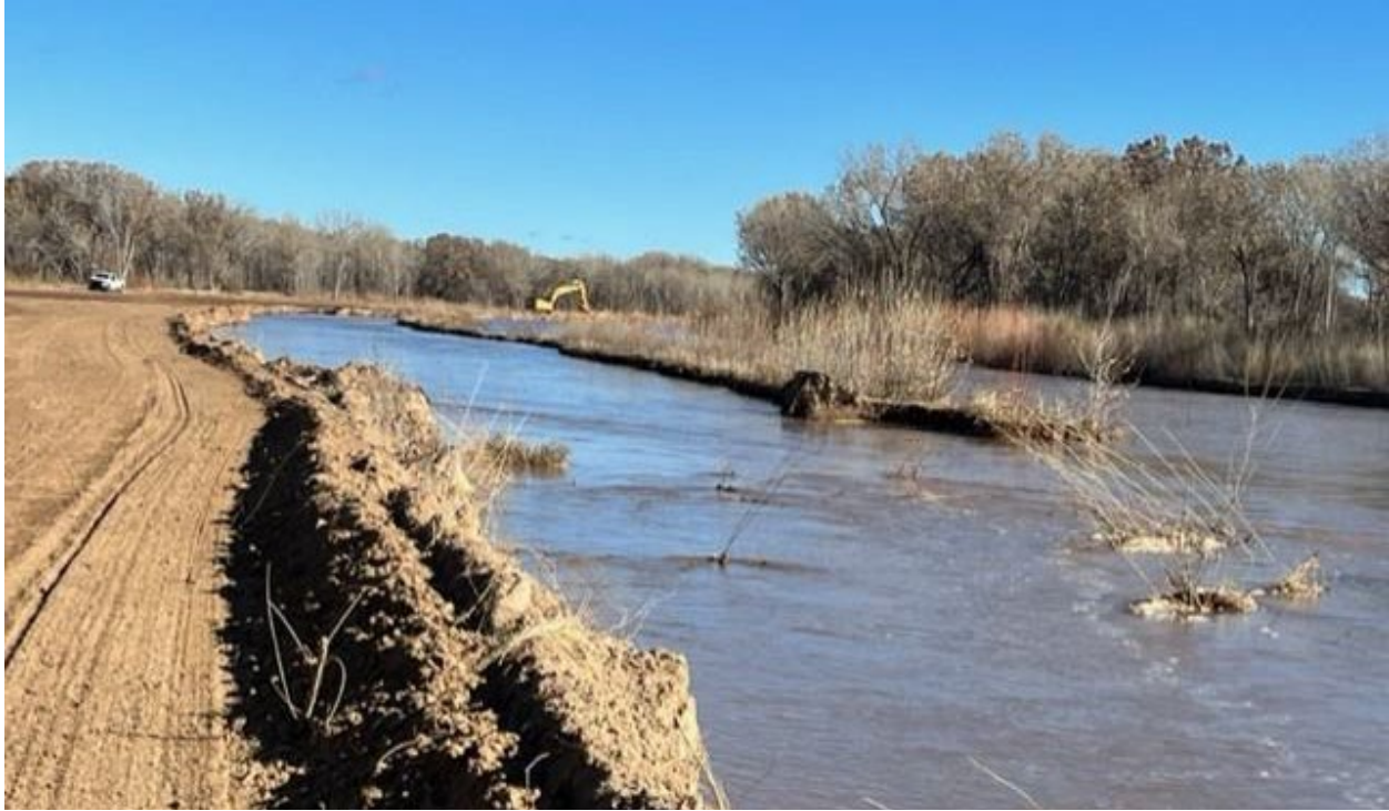
Figure 17: Channel maintenance work at the knickpoint site on the BdA River Realignment Downstream Phase Project (Reclamation, 2023)
