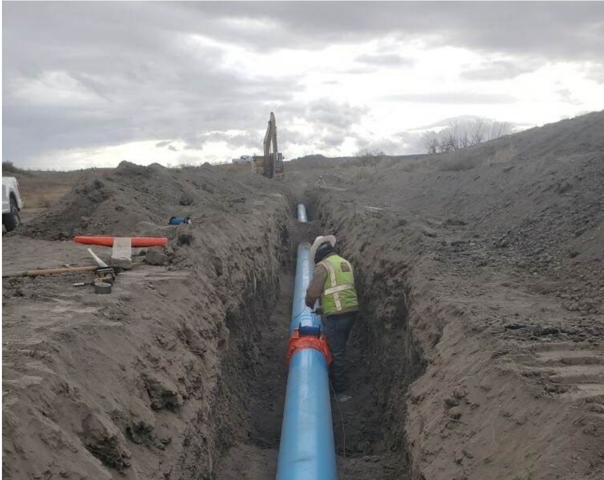
Photograph 1. Example of the pipeline installation process for an irrigation lateral in the Uncompahgre Valley, completed in 2020 (David Bridges, UVWUA).
