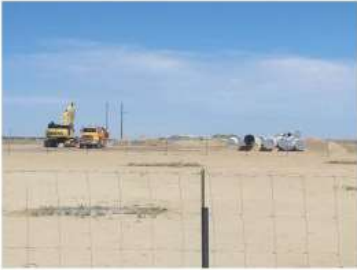
Plastic on end of pipes and littering the range and residential areas
