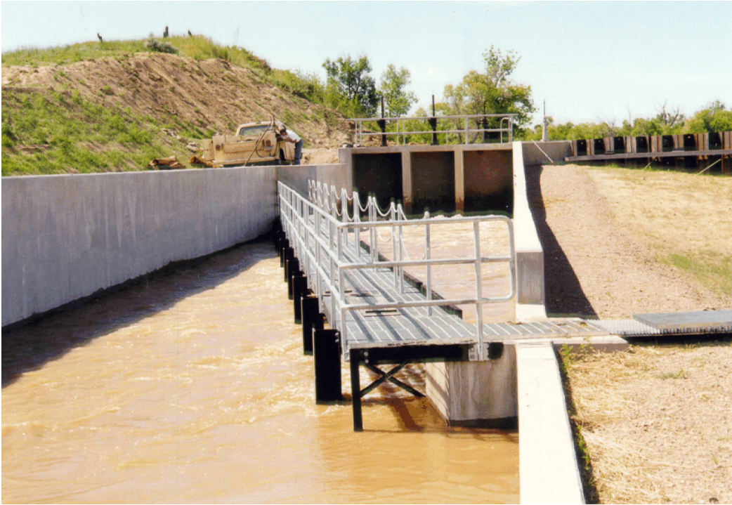
Figure 119.—View looking upstream at the T&Y louver placed at an angle to the canal flow – Example 4 (T&Y Irrigation District).
