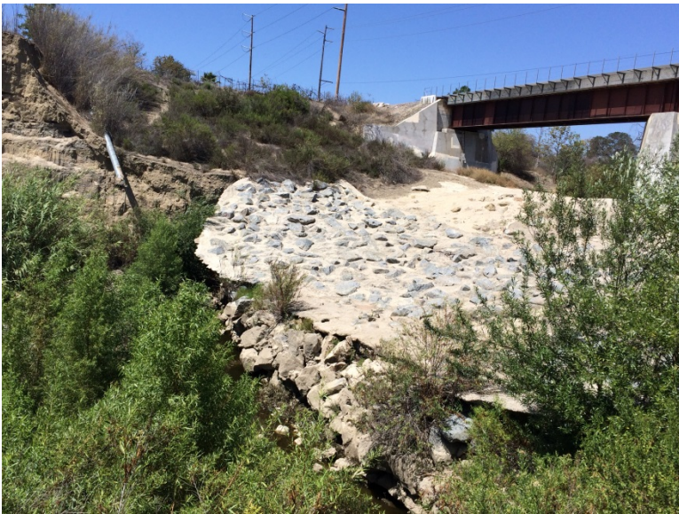
Figure 6. Significant scour hole and stream degradation downstream of the grouted section.
