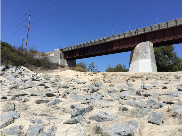
Figure 3. Upstream view of grouted grade control structure at the Metrolink light rail crossing on Trabuco creek.
