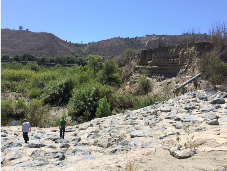
Figure 4. Downstream view of grouted grade control structure at the Metrolink light rail crossing on Trabuco creek.
