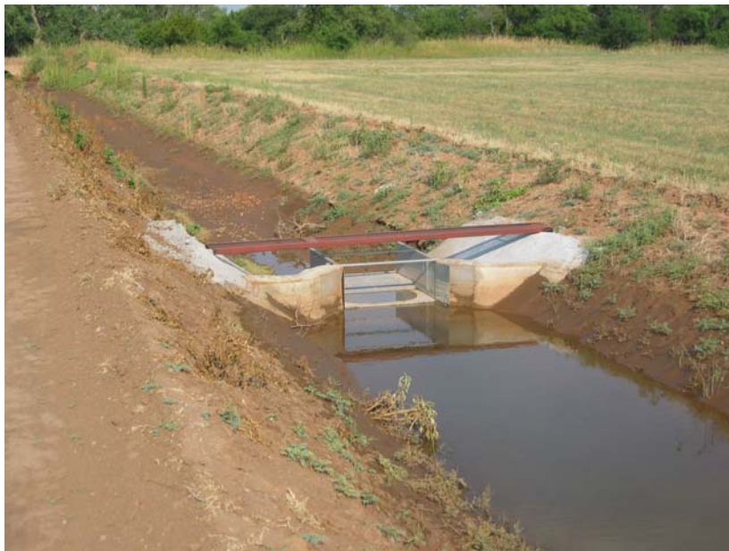
Figure 2. — EZ-Flow flume installed in Ozark wasteway for temporary use in the summer of 2006.
