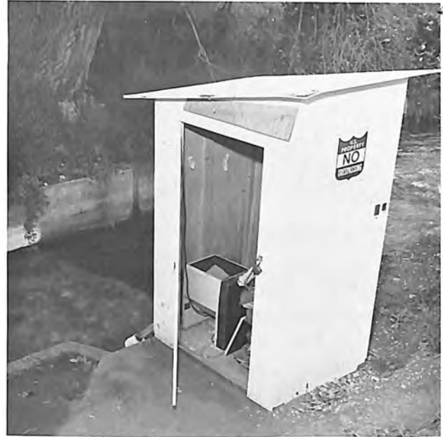
Facilities for feeding copper sulfate into canals include an adjustable-rate feeder with copper sulfate crystals in the hopper and a shelter house to protect the feeder and copper sulfate from weather.
