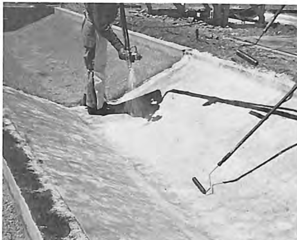
Chopped roving and resin were sprayed on prepared earth canal sections to desired thicknesses, then surface rolled with paint rollers to press the fiberglass into the polyester resin. Seepage losses through this lining were higher than desired.
