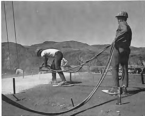
Field test application of pigmented resin base curing- and-bonding compound to a horizontal construction joint surface at Grand Coulee Forebay Dam.
