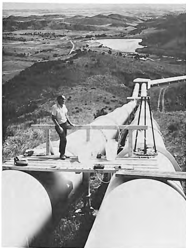
This long penstock leading to Flatiron Powerplant provided an excellent test site for evaluating radioisotopes to measure flow rates in pipelines.
