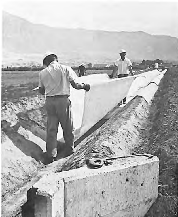
Laminate material for a test lining in a canal is easily installed and is temporarily held in place with steel pins.
