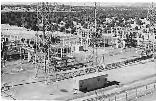
Series capacitor installation at Flagstaff for the two 345-kv Glen Canyon-Flagstaff lines, Colorado River Storage Project. The power system mobile laboratory is in the foreground.
