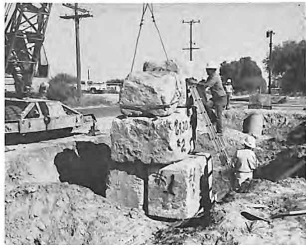
Heavy blocks on a 36-square-foot wooden platform 5 feet above the plastic mortar pipe on compacted backfill produced deflections in the pipe which were measured as part of the installation test program.
