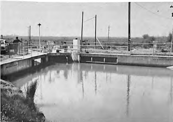
General view looking downstream at the Coyote Creek Check No. 1, Corning Canal. The white cabinet houses the HyFLO controller, which regulates the adjacent check No. 1 gate opening. The primary control signal is received from the hydraulic filter well, located downstream immediately above the next check, a distance of 1.5 miles.
