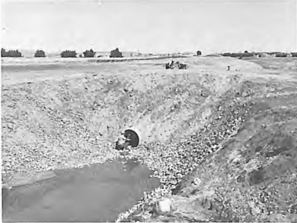
Test section of 48-inch-diameter steel, reinforced plastic mortar and pretensioned concrete pipe under 15 feet of soil backfill at the E&R Center to determine pipe deflections over a period of years.
