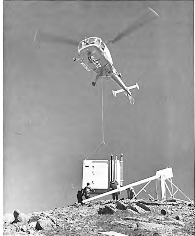
A helicopter delivers material to a remote mountain-top site for construction of an instrumentation station.
