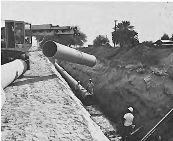
Yuma Project employees laying 30-inch inside-diameter plastic mortar pipe in 20-foot lengths with 3/10-inch wall thickness and bell- and spigot-joints.
