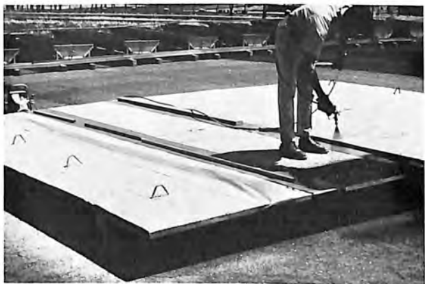
After the vapor-barrier coating has dried on the concrete roof deck, urethane foam will be spray-applied to form a watertight, insulated roofing system.
