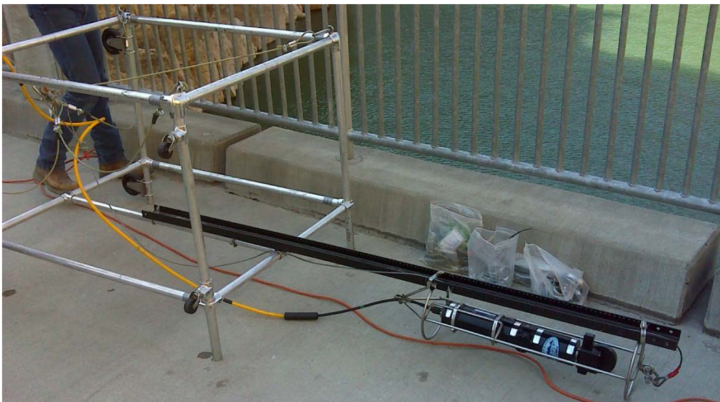
Figure 5. Modified sonar setup used to offset the transducer 8.5 ft from the dam face. This modification was made in an effort to image the upstream face of the trashrack.
