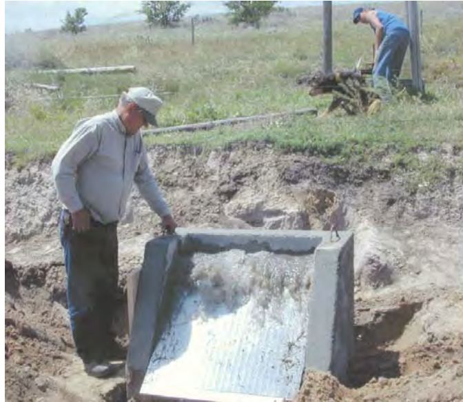
Figure 5. — Coanda-effect screen structure similar to that shown in Fig. 4, operating at a relatively high flow rate. All flow still passes through the screen before reaching the toe.
