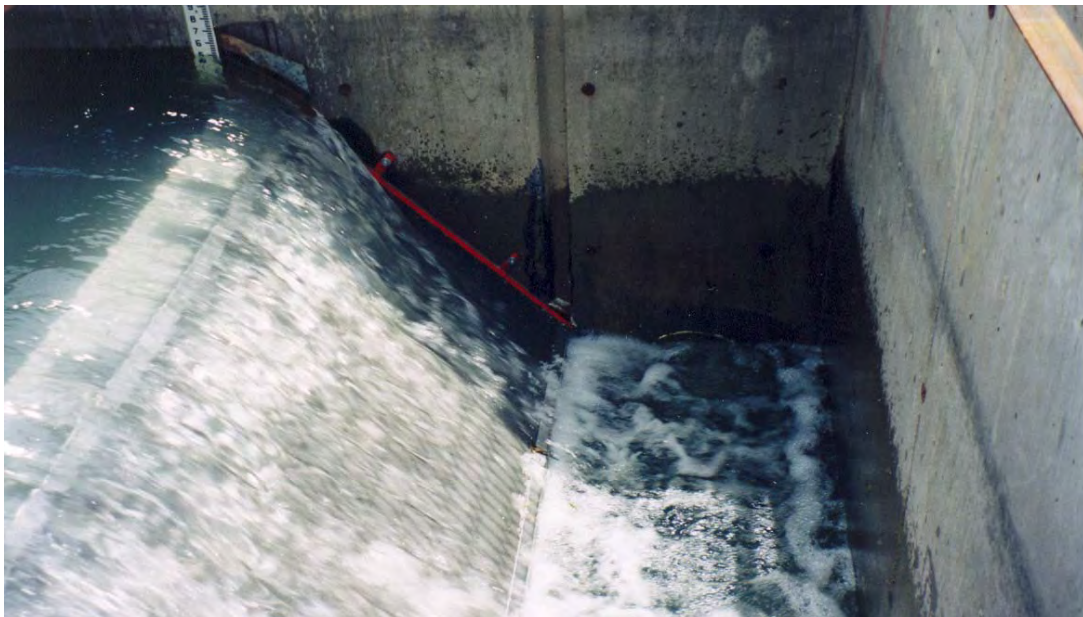
Figure 2. — Coanda-effect screen installed on the Boise Project. Clean water drops through the screen section into a conveyance channel beneath the screen. A staff gage and sheet-metal flow deflector are visible at the upstream corner of the screen.
