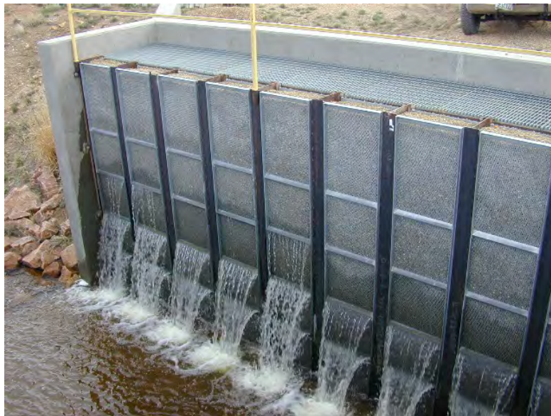
Figure 6. — Sand filter at Lake John. This structure presented some exciting maintenance challenges.
