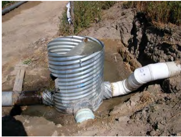
Figure 3. — Coanda-effect screen structure built with corrugated metal pipe. Raw water enters from the right. Clean water is discharged through the center and left-hand pipes, while debris exits onto the ground through the slot in the left side of the structure.
