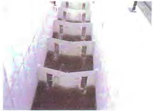
Figure 11 – View looking downstream at the Pyramid Lake fishway dual-vertical slot fish ladder.
