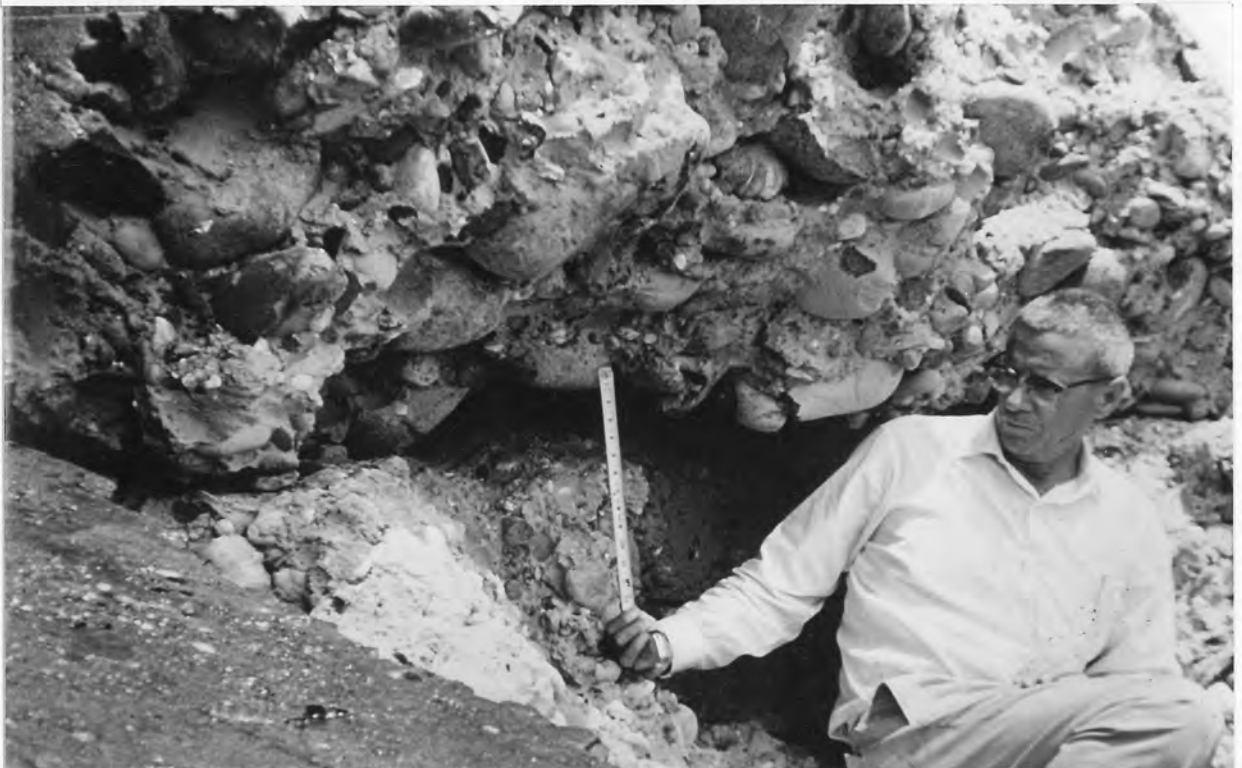
FIGURE 9. CAVITATION EROSION IN CONCRETE AT THE JUNCTION OF OUTLET 7, FOLSOM DAM, CALIFORNIA
