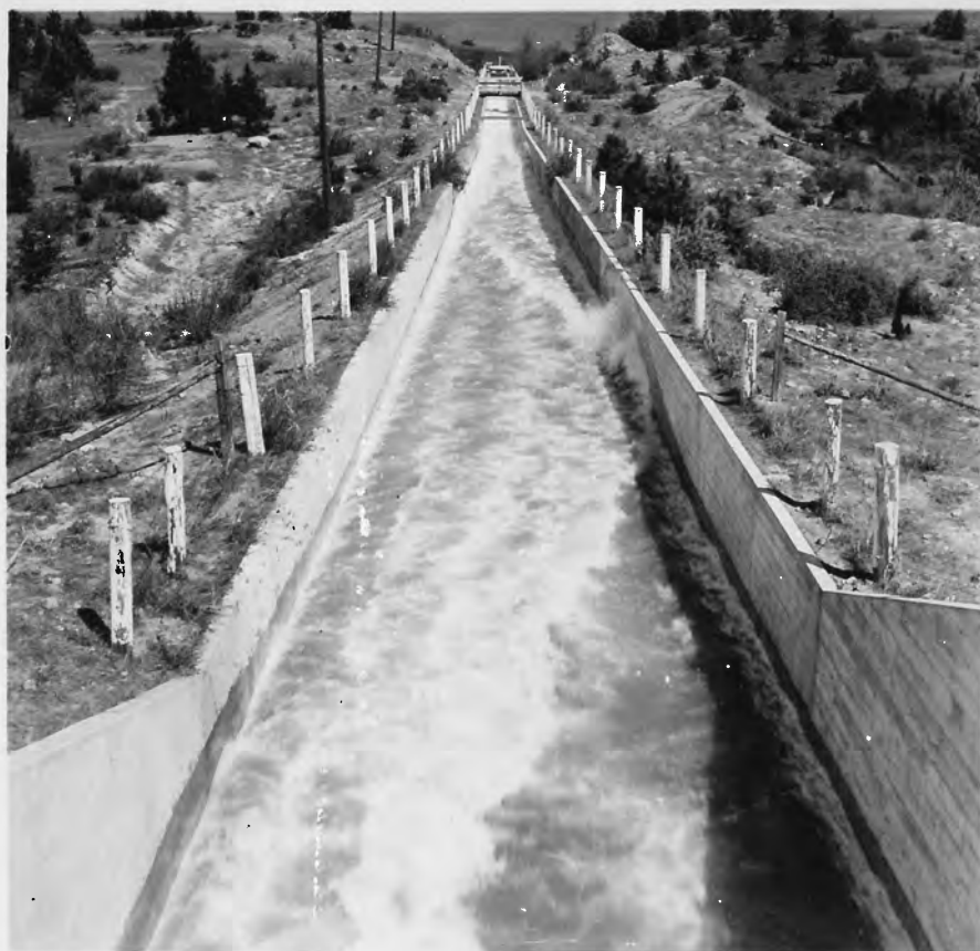
B. WAVE IN UPPER SECTION OF WASTEWAY CAUSED BY ENTRANCE CONDITION. DISCHARGE 922 SECOND-FEET
