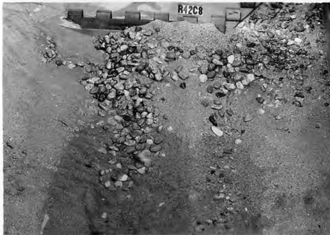
C. SCOUR AT END OF APRON.
