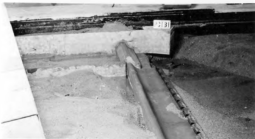
PITS AT LEFT END OF SPILLWAY AND ADJACENT TO THE INTAKE WORKS.
