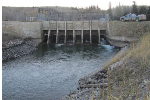
Figure 5. St. Mary Diversion headworks structure (the view is from downstream of the headworks, with flow towards the reader).
