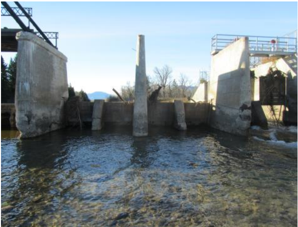
Figure 8. Concrete degradation on the downstream end of piers surrounding sluice bays.
