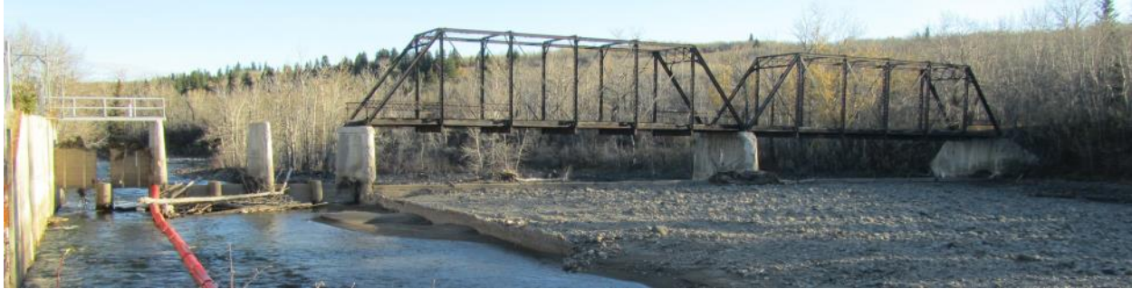
Figure 3. Existing St. Mary Dam Diversion weir, sluiceway and abandoned bridge during low flow fall season (the view is from the upstream left bank).
