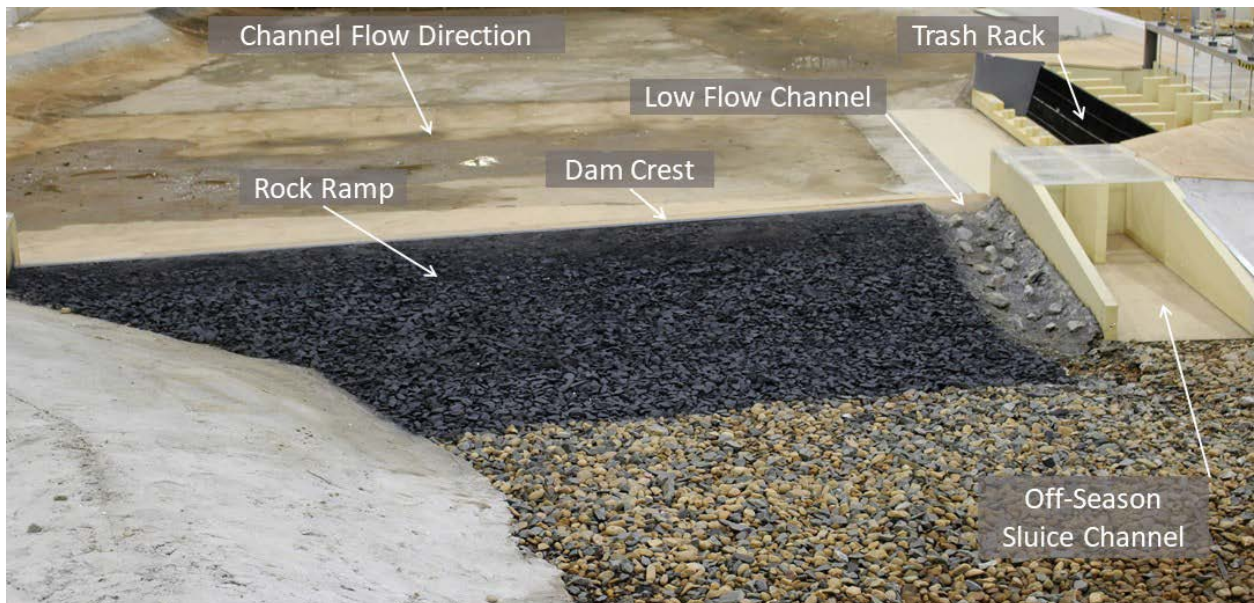
Figure 21. Rock ramp, low flow channel, off-season sluice, dam crest and trashrack (the view is from the downstream middle of river channel).
