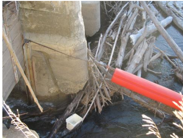
Figure 9. Concrete degradation on the upstream sluice bay pier noses.
