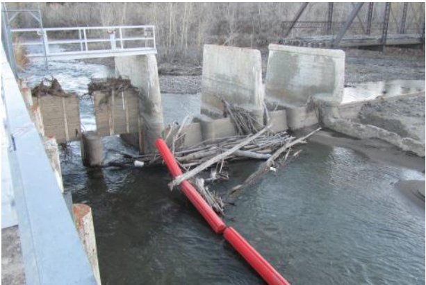
Figure 4. St. Mary Diversion sluiceway gates (the view is from the upstream left bank, standing on top of the headworks structure).
