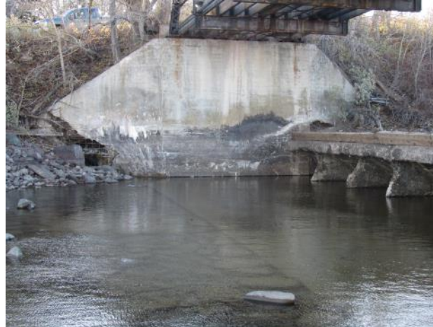
Figure 7. St. Mary Diversion right abutment damage and exposed rebar.
