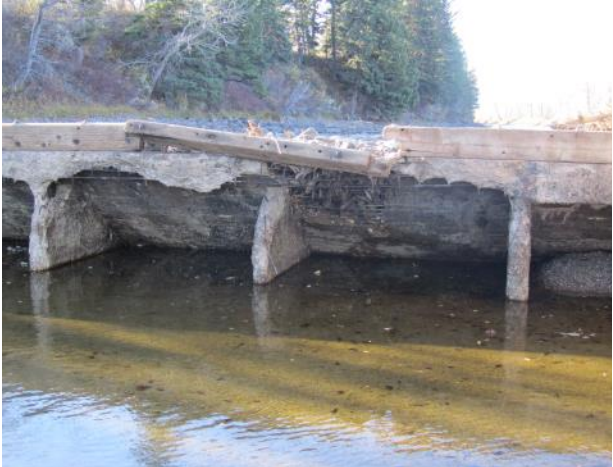
Figure 6. St. Mary Diversion weir concrete failure and exposed rebar.
