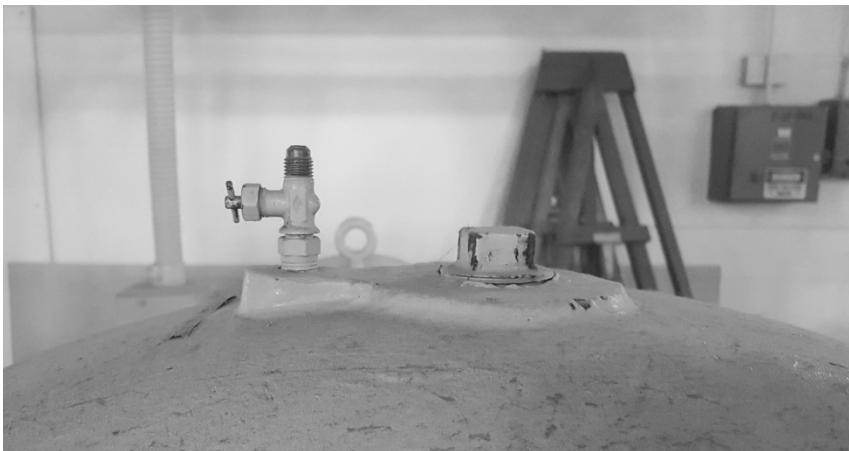
Figure 20: Bleed valve on top of main pump casing. This valve can be closed once the air has been forced out of the pump by the rising water.
