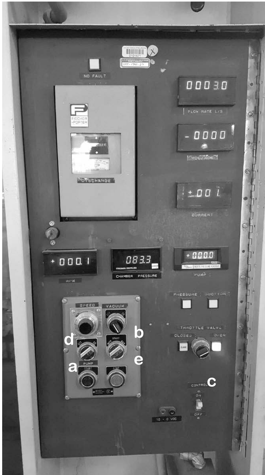
Figure 13: Main control panel for LAPC at the top of the stairs.
