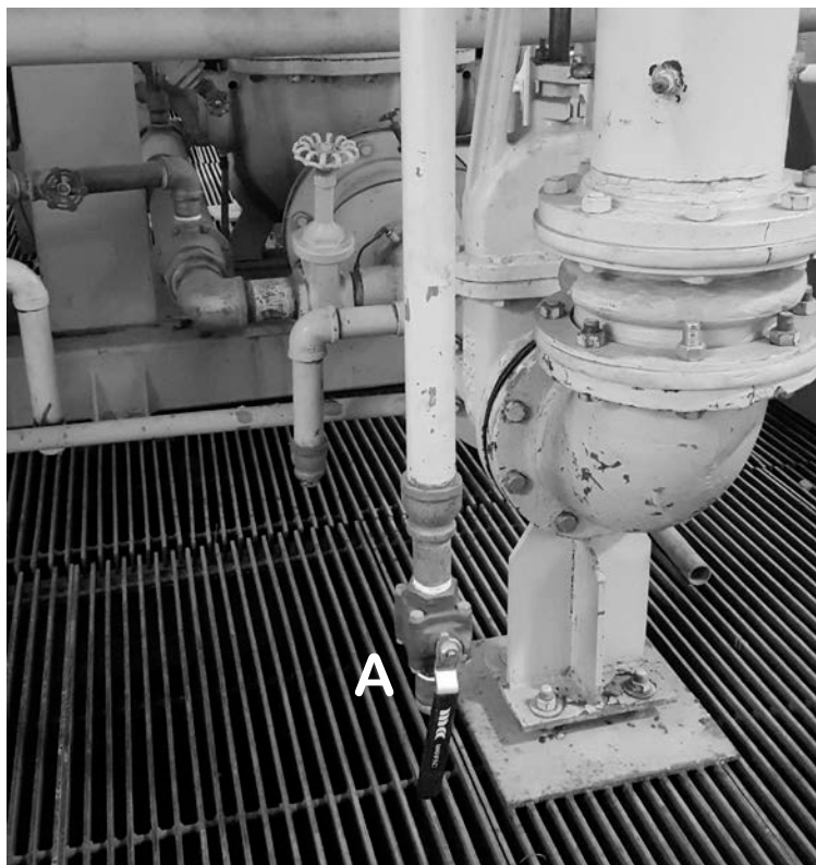
Figure 5: North end of LAPC, chamber drain piping, A) drain valve.
