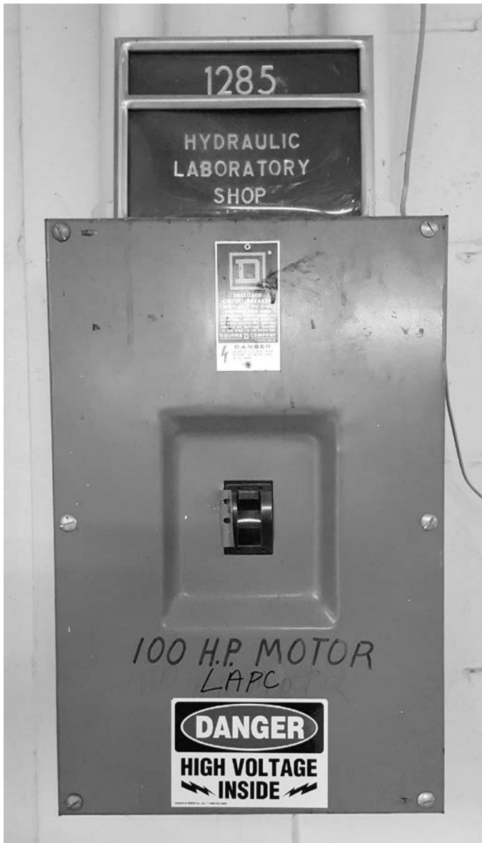
Figure 9: Remote shutoff for LAPC main motor, located near laboratory shops north door.
