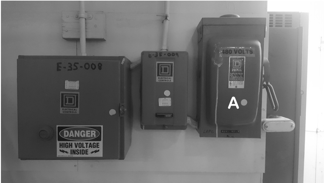
Figure 10: Breakers located directly behind the LAPC.
