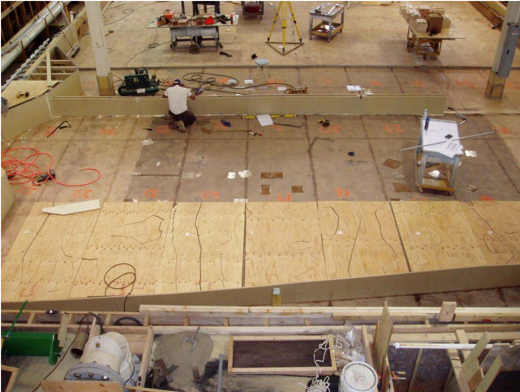
Figure D- 1. Initial phase of model construction of diversion weir and upstream topography.
