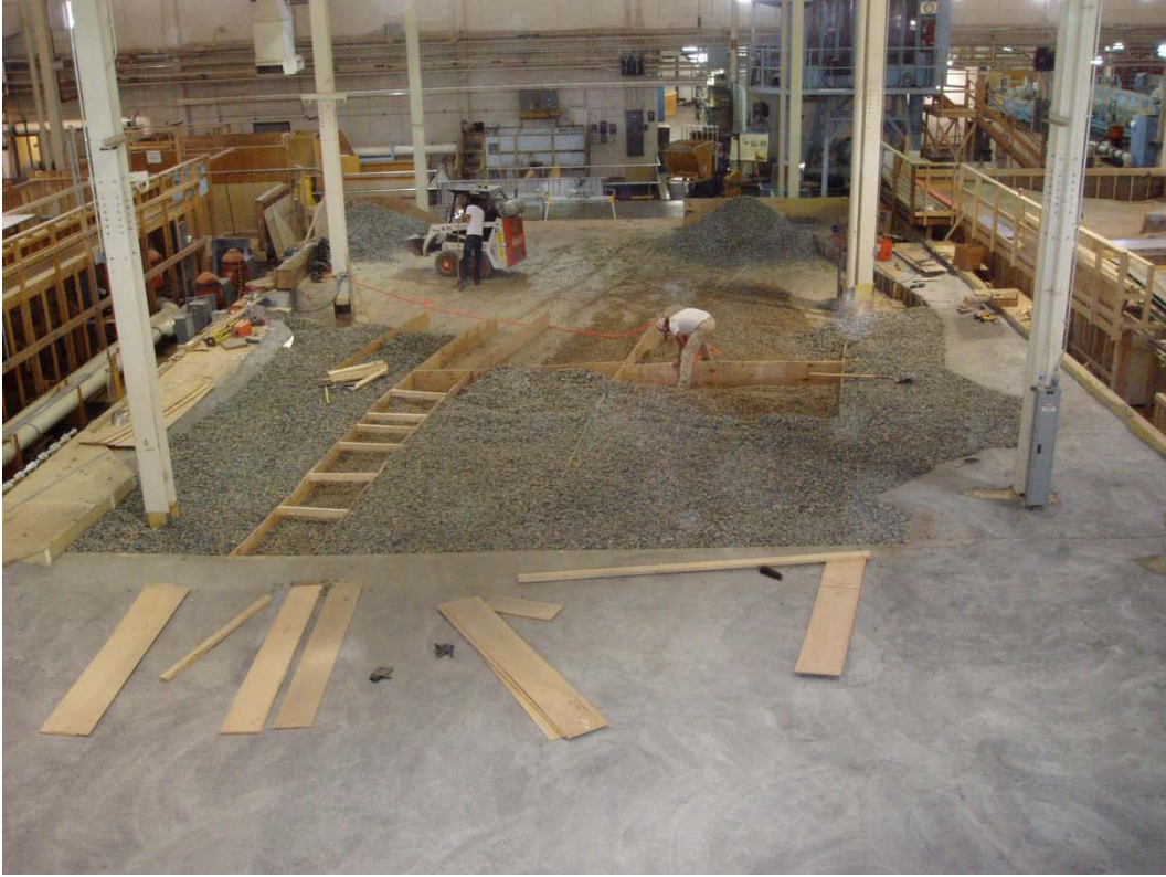
Figure D- 4. Installation of angular rock and breakline templates for model rock ramp.
