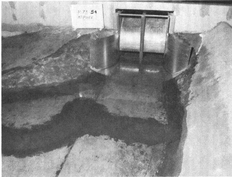
a. Short curved guide walls, radius = 15.24 m (50 ft), leading to spillway. Photo P801-D-79452
