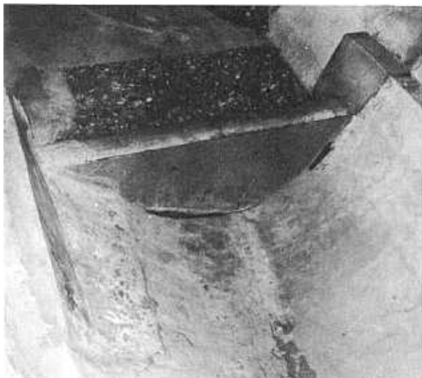
FIGURE 27.—View downstream showing the piers removed from each side of the weir and extension of the lining downstream from the stilling basin.
