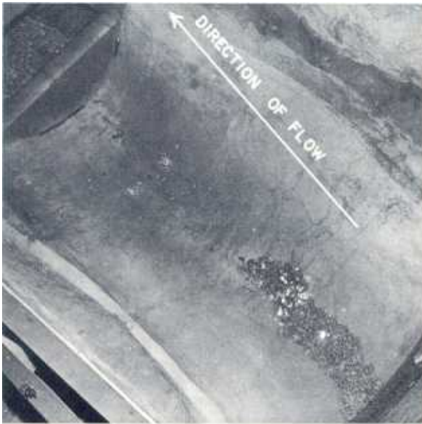
FIGURE 36.—Evidence of rock movement in stilling basin pool after 1 hour at spillway Q=34,400 cubic feet per second. (Maximum design discharge for spillway.)
