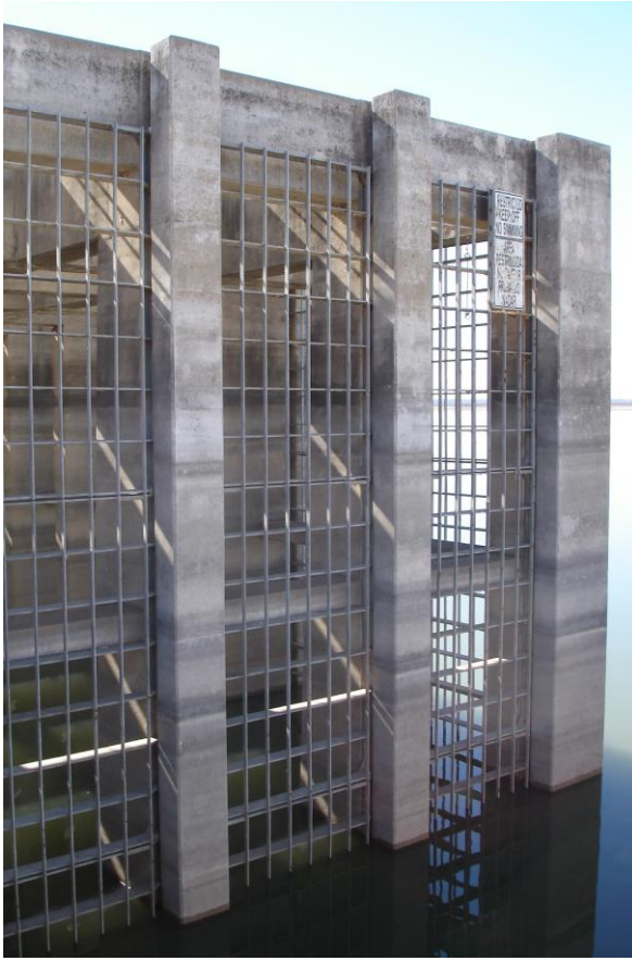
Figure 12.2.1.2-1. Side bearing trashracks at reservoir outlet structure. Note the vertical, stacked trashrack panels installed within the concrete structure grooves (slots).
