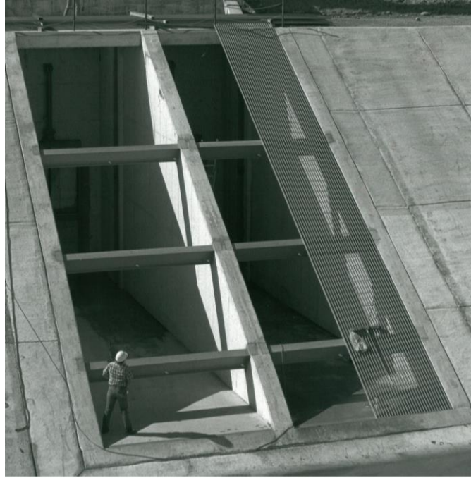
Figure 12.2.1.1-2. End bearing trashracks with horizontal support beams being installed at canal turnout intake.
