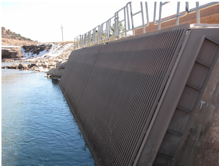
Figure 12.2.1.2-2. Side bearing trashracks at river side intake. Note the inclined trashrack panels installed within metal trashrack side guides.
