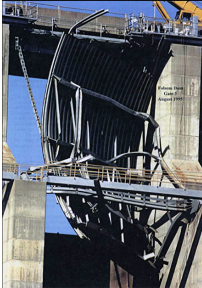
Figure G-1-3.—Failure of radial gate No. 3 at Folsom Dam.
