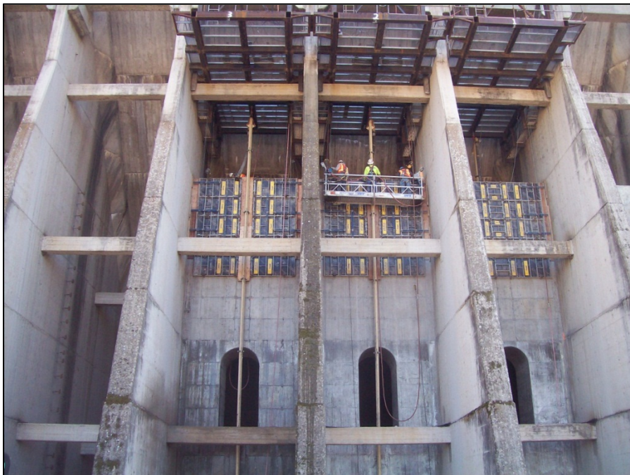
Figure 1 - View looking upstream. Three arched and three solid diaphragm walls shown. Formwork installed on three additional diaphragm walls above. Stony Gorge Dam Modification.
