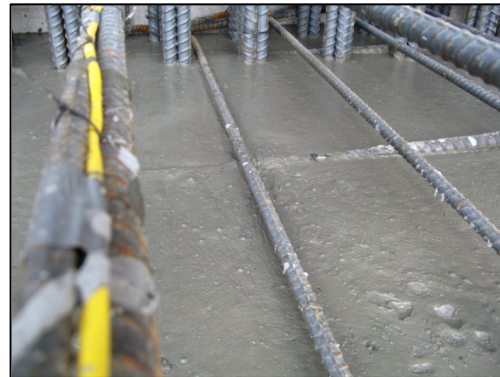
Figure 20 - Six-inch slump high strength RSMC nearing temperature instrumentation wires. Deer Creek Dam Spillway Modification.
