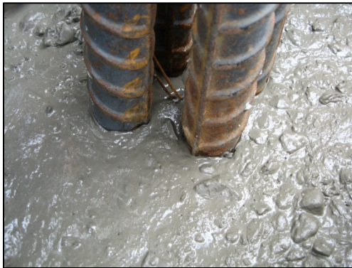
Figure 19 - Six-inch slump high strength RSMC flowing through bundled No. 11 reinforcing steel bars. Spacers were placed between the bars to allow concrete to fill in the void. Deer Creek Dam Spillway Modification.
