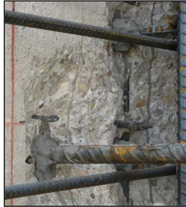
Figure 33 - Cleanup of left counterfort wall surface prior to placement of the RSMC. Deer Creek Dam Spillway Modification.
