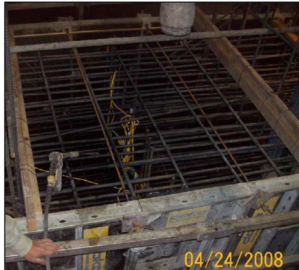
Figure 4 - Diaphragm wall prior to concrete placement with temperature sensors installed (yellow wire). Stony Gorge Dam Modification.
