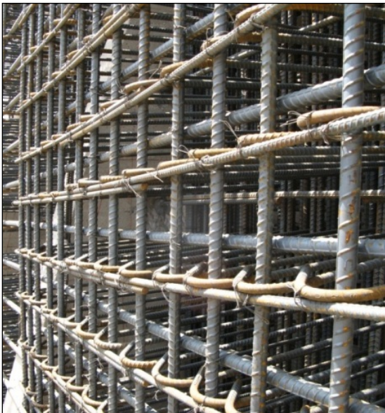
Figure 12 - Reinforcing steel for left seismic wall buttress. Deer Creek Dam Spillway Modification.
