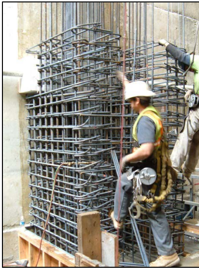
Figure 3 - Diaphragm wall reinforcing steel prior to formwork installation. Stony Gorge Dam Modification.
