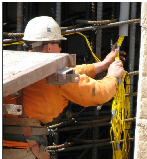
Figure 16 - Bundled lead wires being routed into 2 in. diameter pipe. Deer Creek Dam Spillway Modification.
