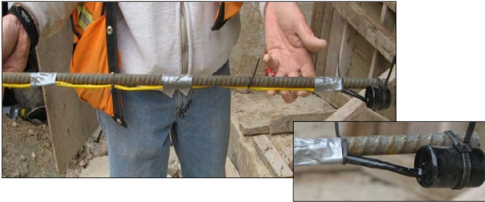
Figure 13 - Temperature sensors attached to reinforcing steel ready for placement in the left seismic buttress wall. Deer Creek Dam Spillway Modification.
