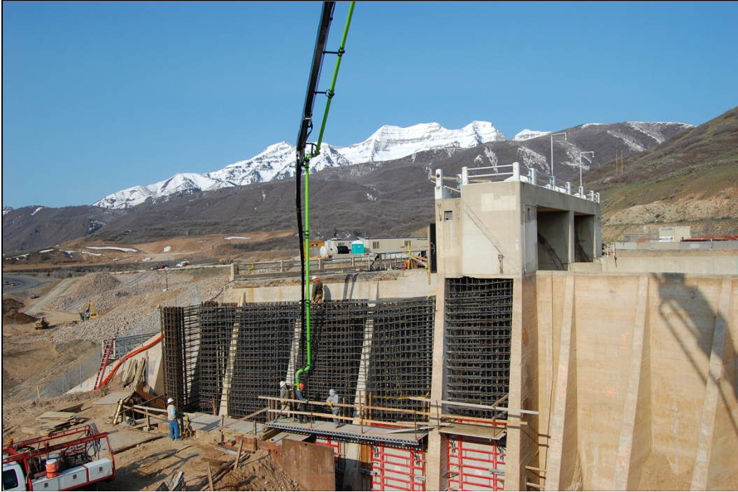
Figure 9 - RSMC seismic buttress encases the original left spillway wall counterforts. Deer Creek Dam Spillway Modification.
