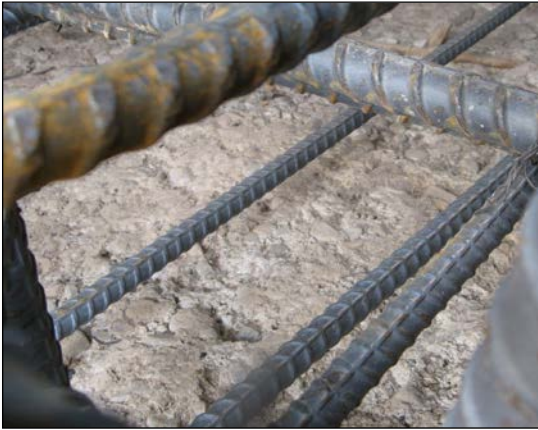
Figure 32 - Construction joint lift surface cleanup for RSMC. Deer Creek Dam Spillway Modification.
