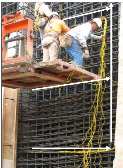
Figure 15 - Installation of temperature sensors and wire leads. Deer Creek Dam Spillway Modification.
