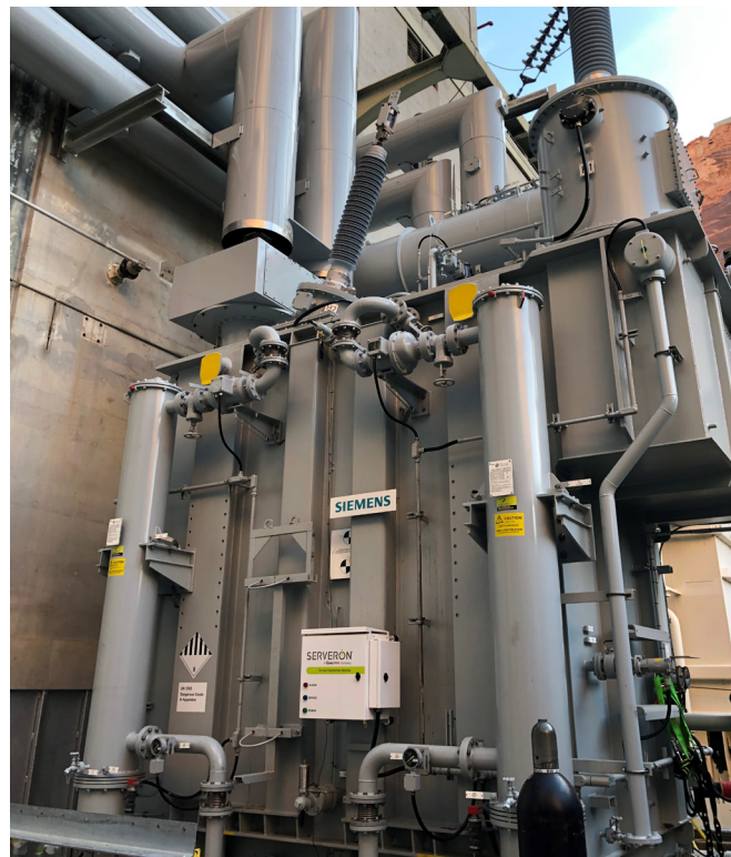
Natural ester fluid (FR3) power transformer at Glen Canyon Dam.
