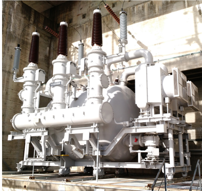
Gas insulated (SF6) power transformer at Osage Power Plant.
