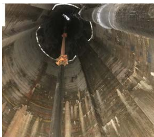
Image showing the physical dryness of the walls.
