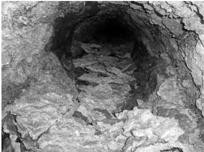
Figure 1. Pipeline scaling of highly concentrated brine lines (Santa Ana Watershed Project Authority, 2010).
