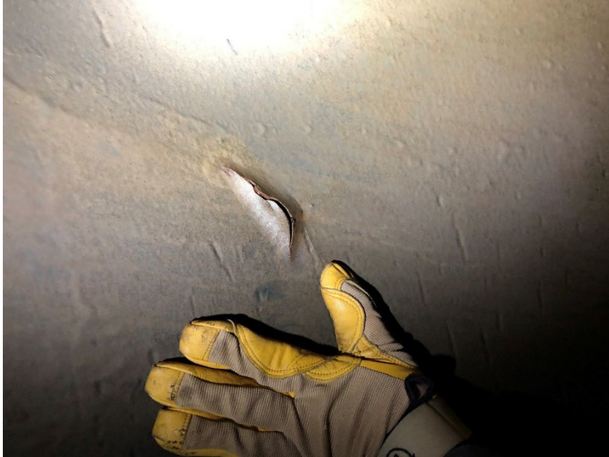
Photo 34. Crack that contains undercutting
