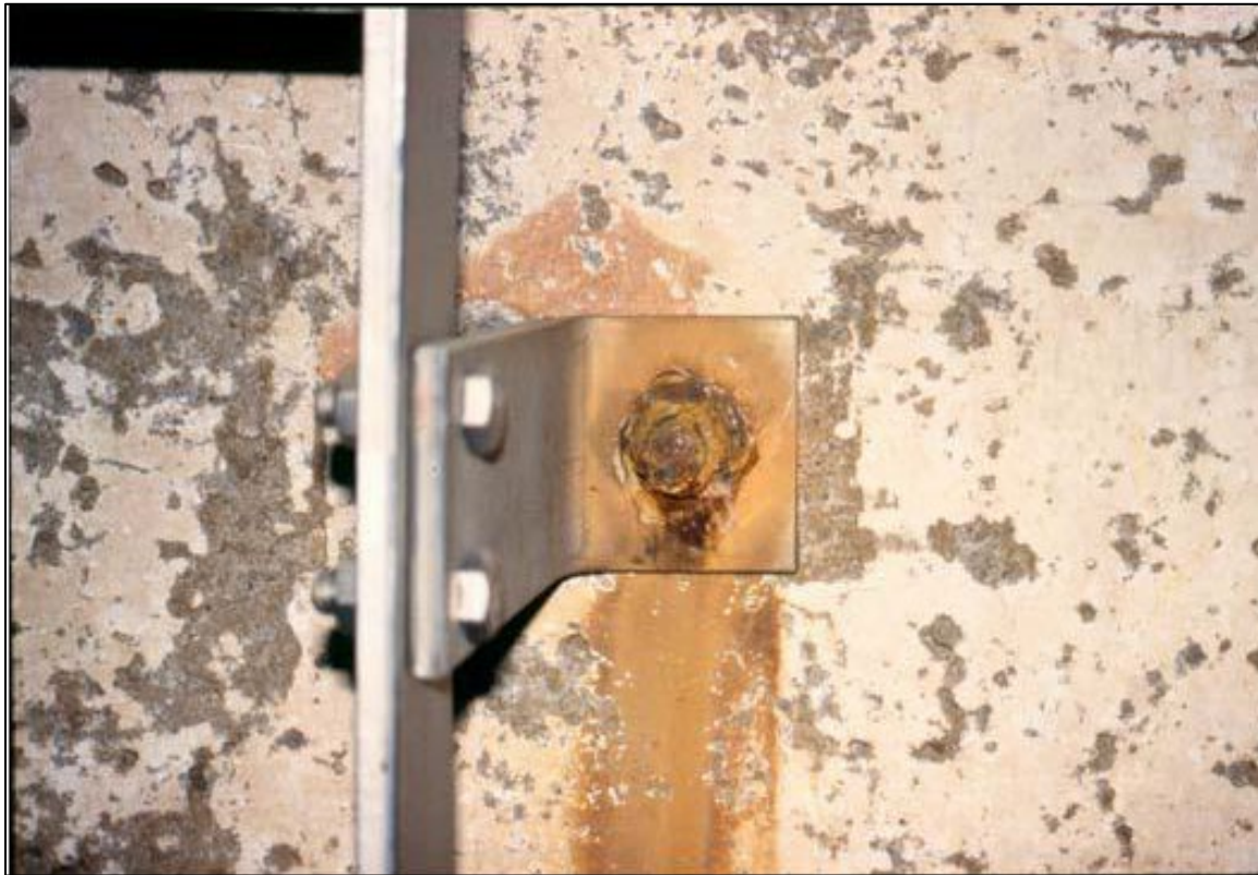
Photo 9. A steel fastener holding a stainless steel ladder demonstrates undesirable anode (fastener) to cathode (ladder) area ratio
