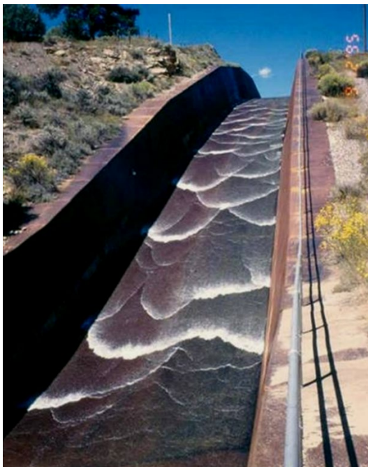
Photo 1. General corrosion on a spillway
