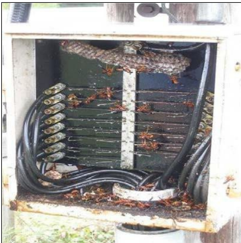
Photo 39. Wasps occupying a junction box
