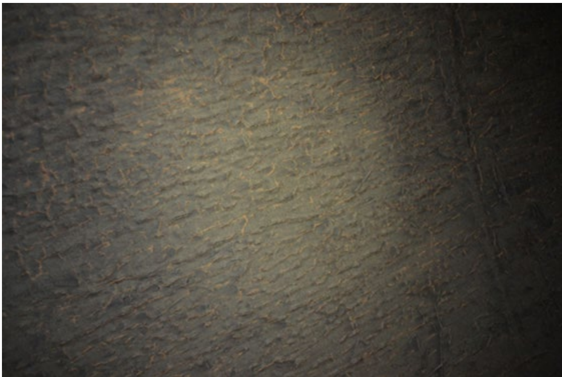
Photo 17. Field representation of stage 5 alligator cracking with undercutting
