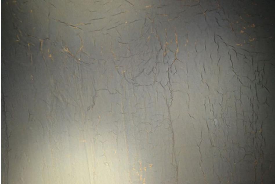
Photo 14. Field representation of stage 3 alligator cracking
