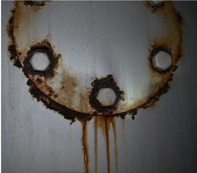
Photo 4. Crevice corrosion on a radial gate access port
