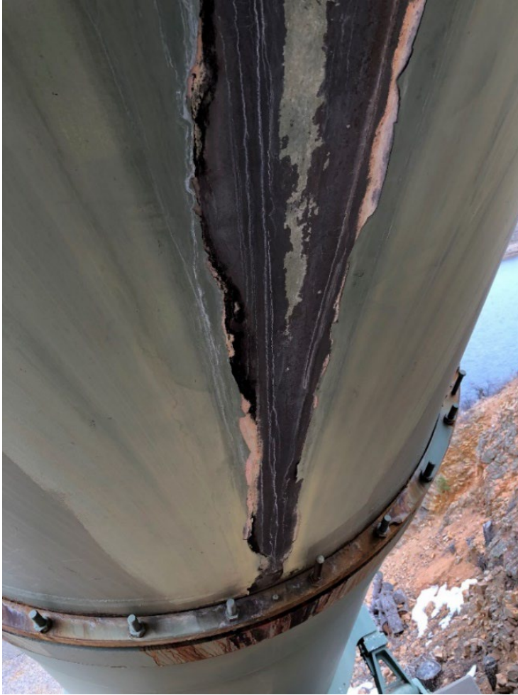
Photo 24. Peeling coating on penstock exterior
