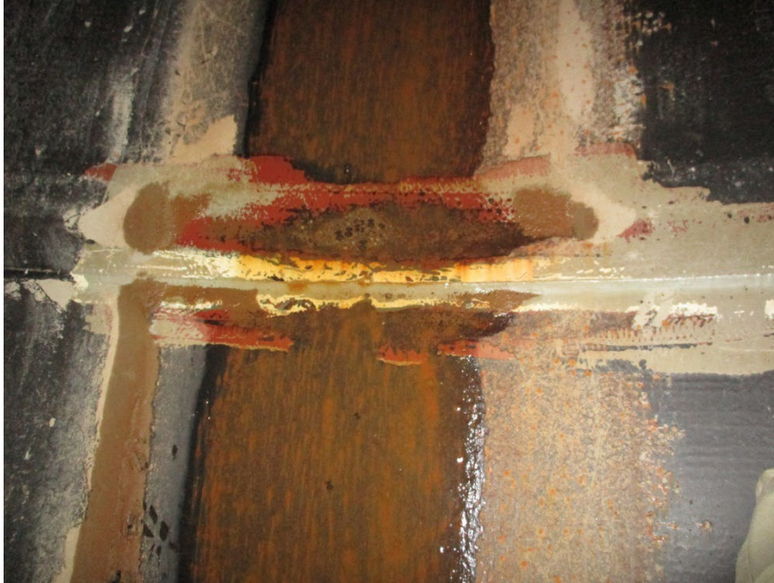
Photo 29. Eroded coating at a pipe joint
