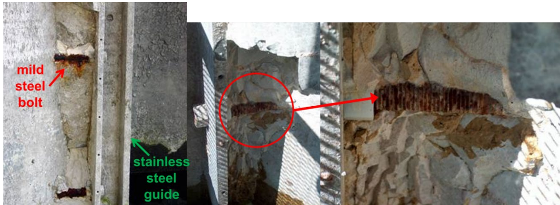
Photo 2. Galvanic corrosion of a mild steel anchor bolt due to the stainless steel stoplog guide
