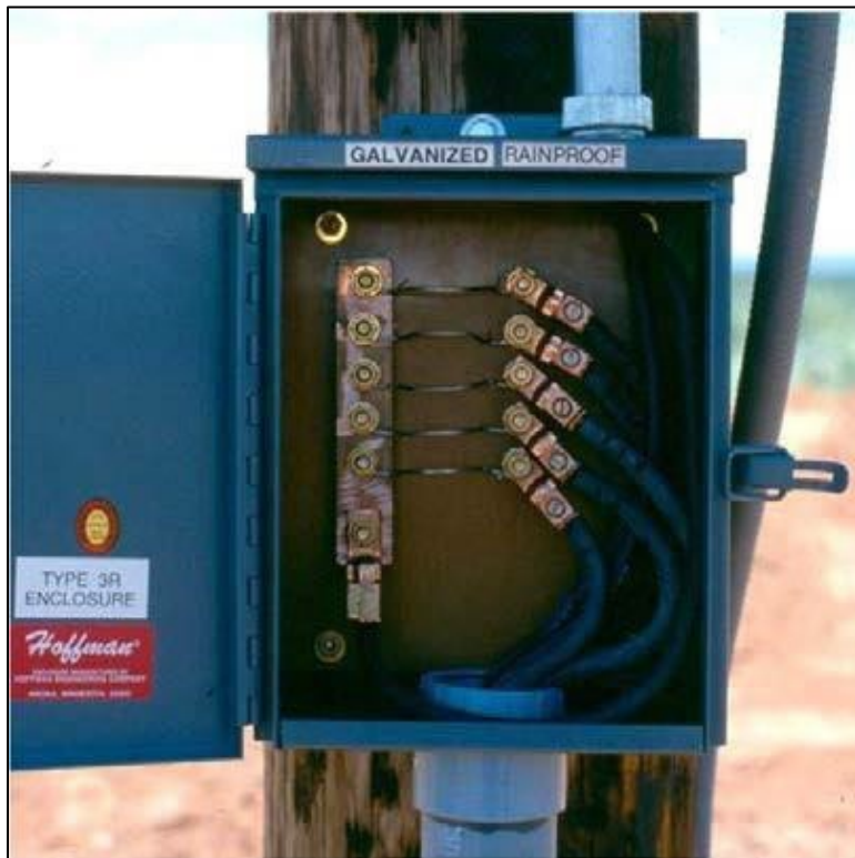
Photo 42. Typical junction box
