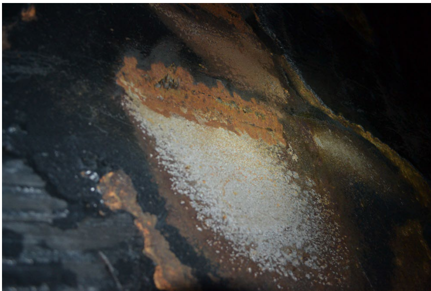
Photo 21. Close up view of cavitation damaged lining
