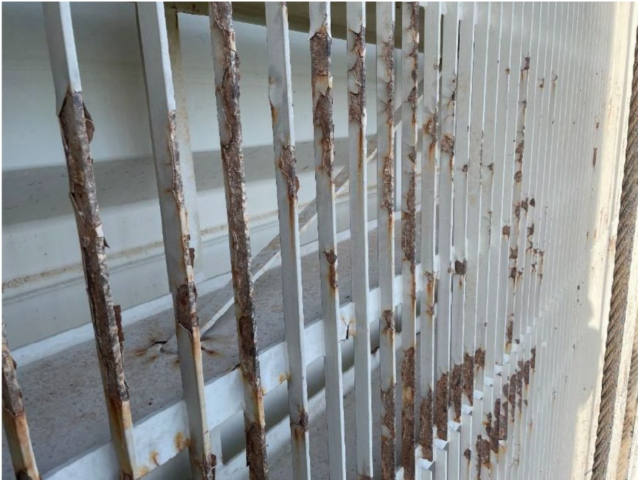
Photo 25. Spalling and missing coating of trashrack structure
