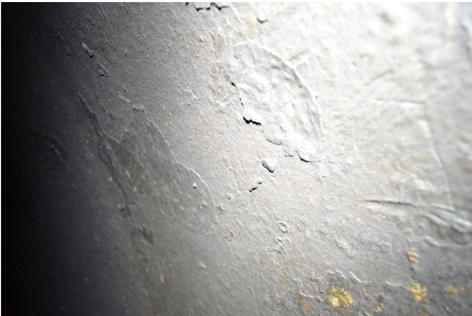
Photo 26. Flaking topcoat on pipe lining
