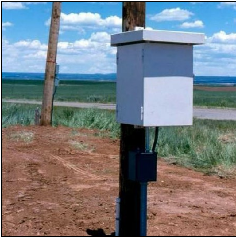
Photo 37. Typical rectifier cabinet
