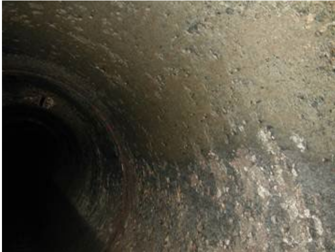
Photo 5. Pitting of the interior of the outlet works pipe
