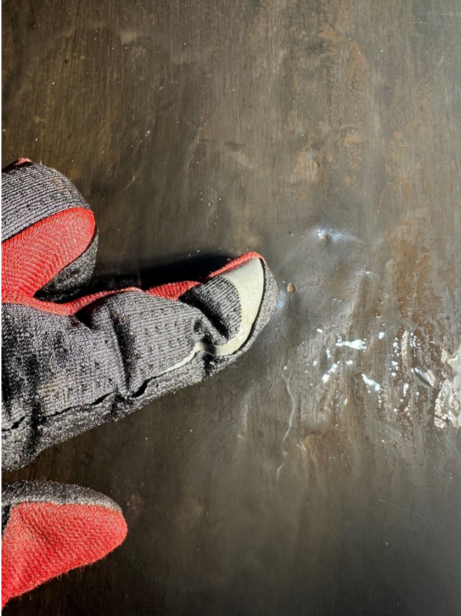
Photo 31. Pinhole in a coal tar enamel penstock lining
