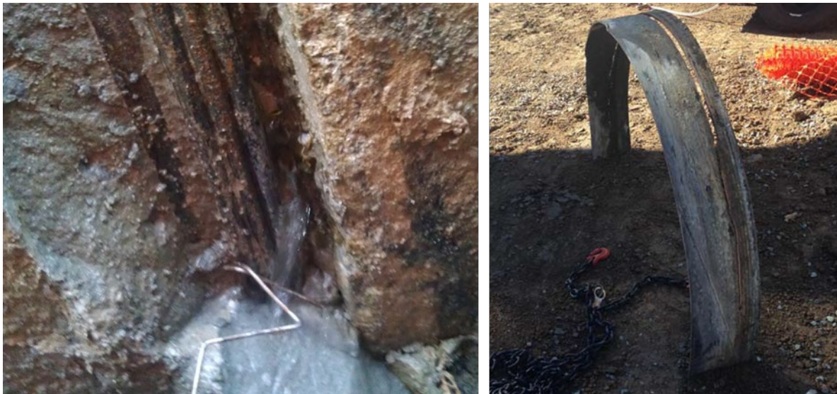
Photo 8. Stress corrosion cracking of a steel bell and spigot joint on a pretensioned pipe
