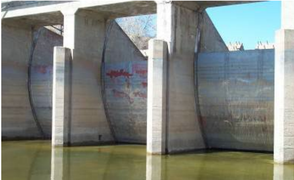
Photo 11. Abrasion damage from floating debris
