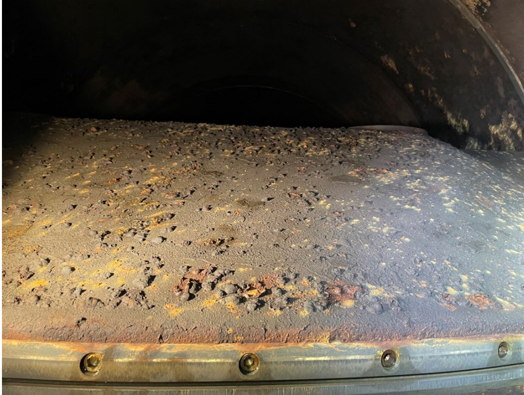
Photo 33. Rust nodules on butterfly valve that is heavily corroded
