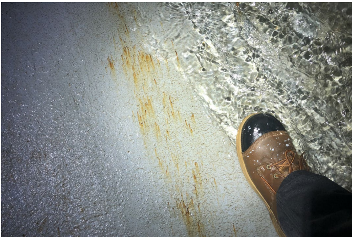
Photo 32. Pinholes in vinyl lined scrollcase
