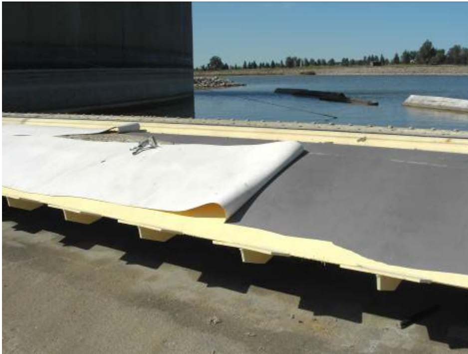
Photo 27. Disbonded coating on spillway gate
