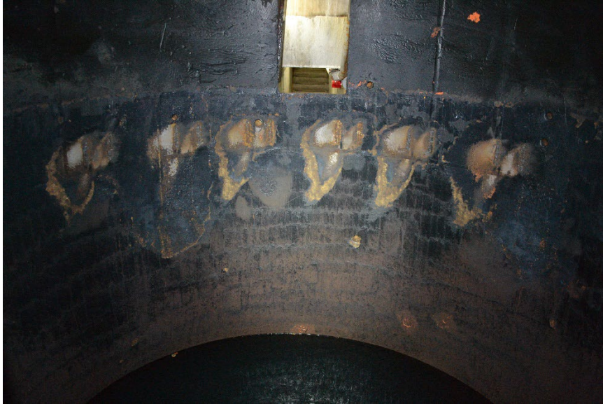
Photo 20. Eroded away lining to steel substrate from cavitation
