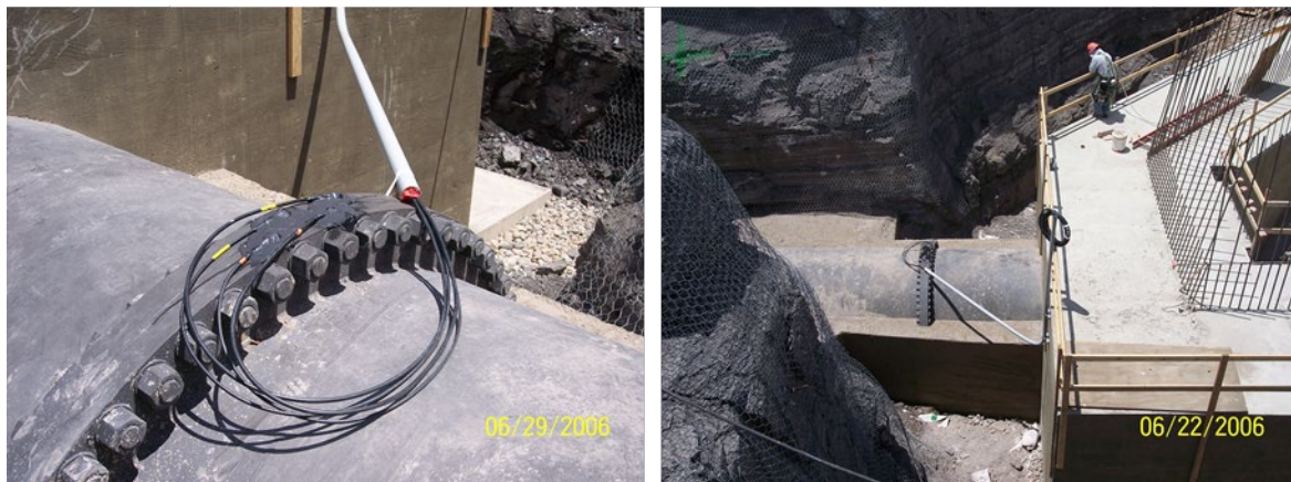
Photo 10. Isolating joints flange kit used to prevent galvanic corrosion of the buried steel pipe
