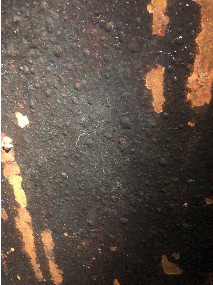
Photo 19. Irregular shaped blisters in coating
