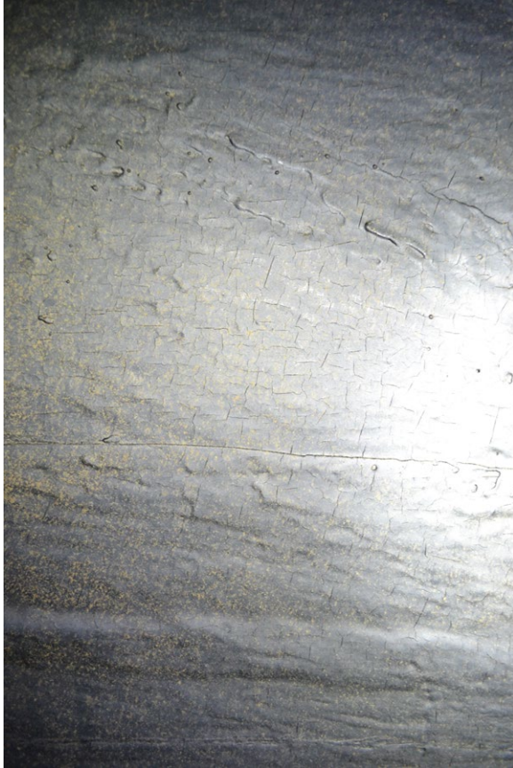
Photo 12. Field representation of stage 1 alligator cracking
