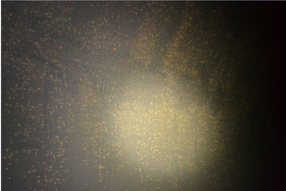
Photo 16. Field representation of stage 5 alligator cracking
