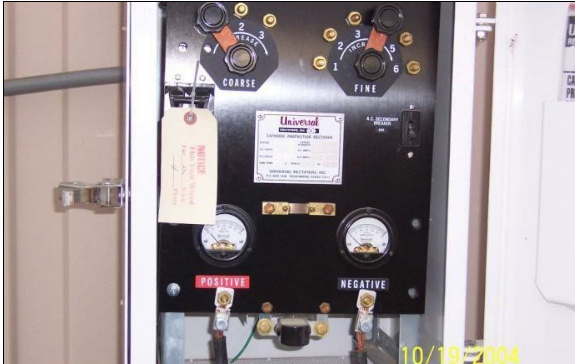
Photo 38. Typical rectifier board inside a cabinet
