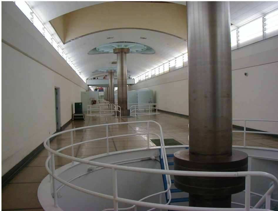
Photo 14.—Shaft and coupling.
