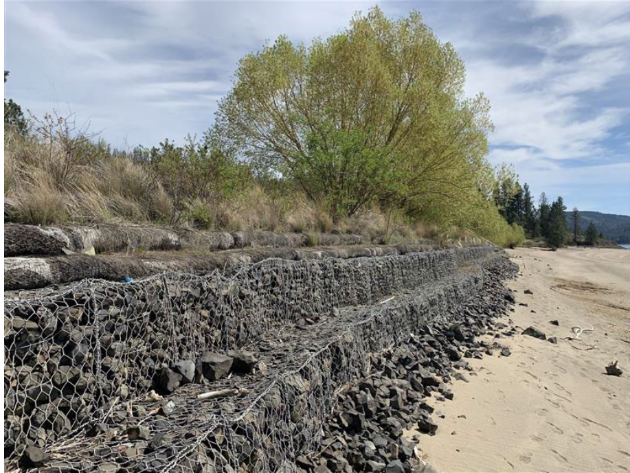
Figure 2-2. Example of gabions baskets used at a Reclamations Lake Roosevelt shoreline stabilization project.
