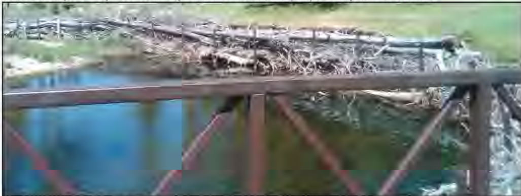
An undersized bridge on Hole 6 – the pier 3. The logs piled horizontally are hand-placed aimed at stopping the severe cut-bank erosion just downstream from the bridge. Just upstream from the bridge has been incised by the narrowing of the river.
