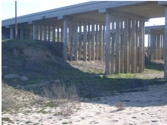
Figure 3-12. Erosion in Bypass Channel at SH 152
