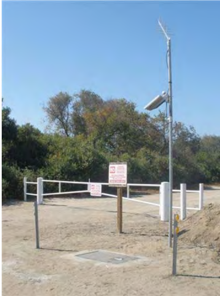
Figure F- 5: Real-time monitoring well
