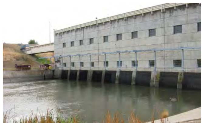
C.W. "Bill" Jones Pumping Plant (formerly Tracy Pumping Plant)
