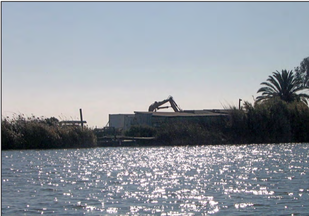
Photo 16. This photo also depicts the heavy equipment present within the marsh used for maintenance activities.
