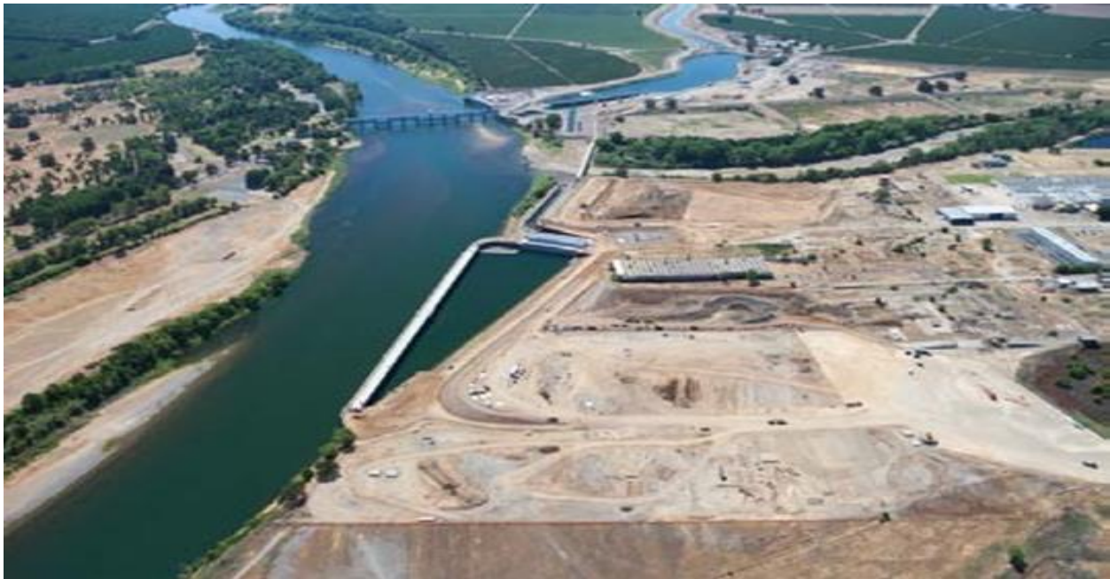
Figure A-23. Picture of Red Bluff Pumping Plant
