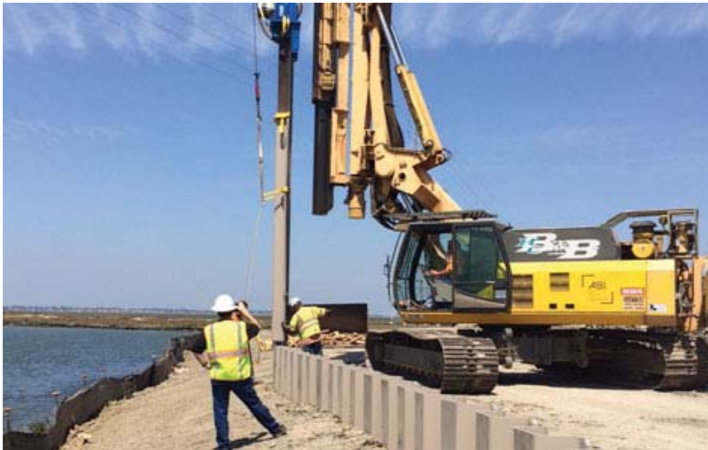
Figure V-9.—Example of track-mounted, fixed-mast vibratory hammer equipment that would be used for the sheet pile installation. (CMI Shoreguard)
