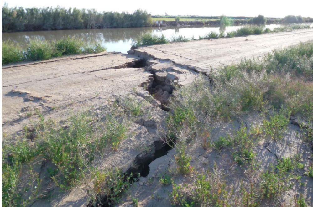
Figure VI-1.—Example of Seismic Related Embankment Cracking, All American Canal Lateral, 2010.
