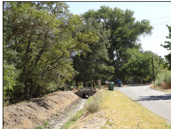
Figure 4. Looking east down the TC-1-1 lateral canal to the box culvert and private road crossing for the proposed pipeline.
