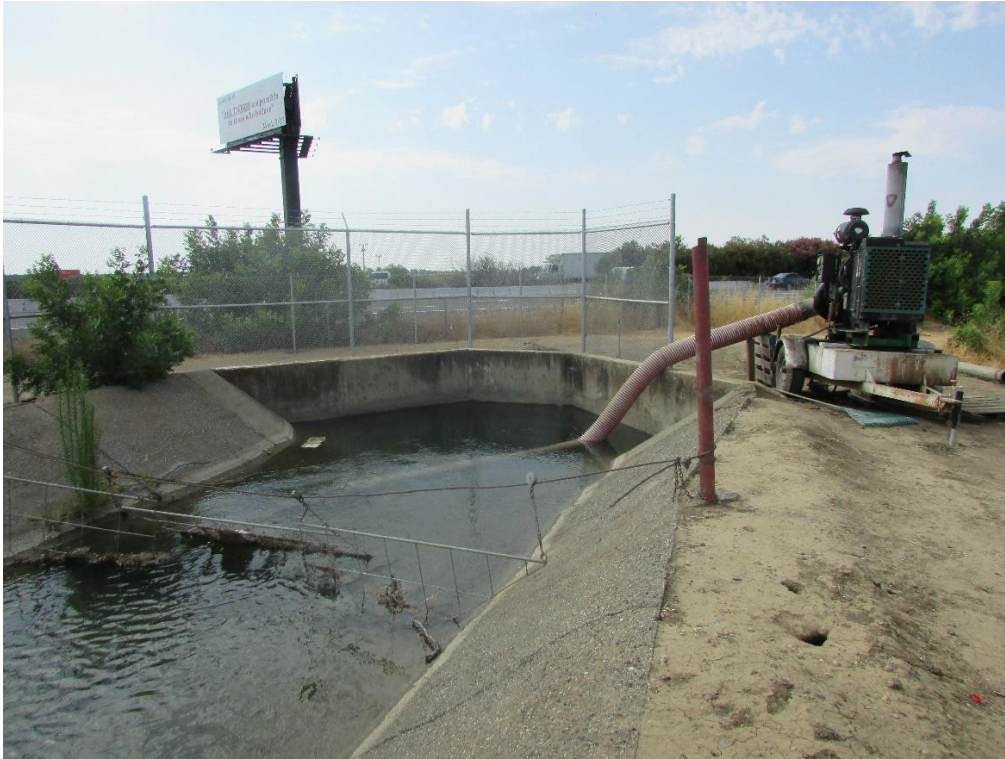
Representative Photograph 1. Lateral/Turnout #1 and Pump Station #1
