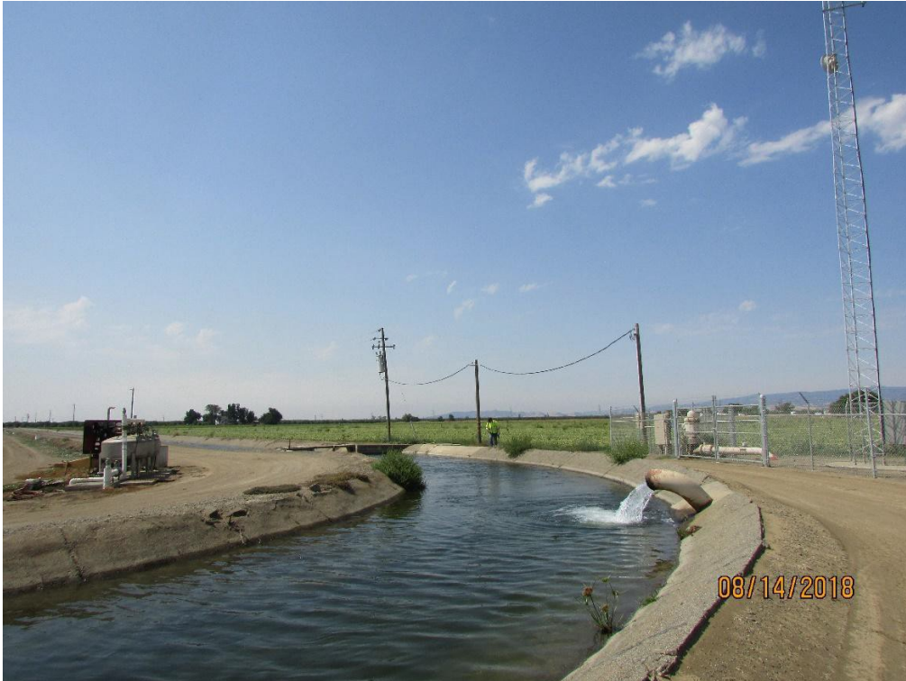
Representative Photograph 4. Lateral/Turnout #4, Check Structure #2, and Pump Station #2.
