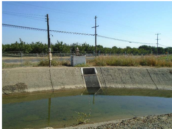
Photo 3. View of the Lateral C headworks of the Weyand Canal from Dixon Avenue, facing northeast.
