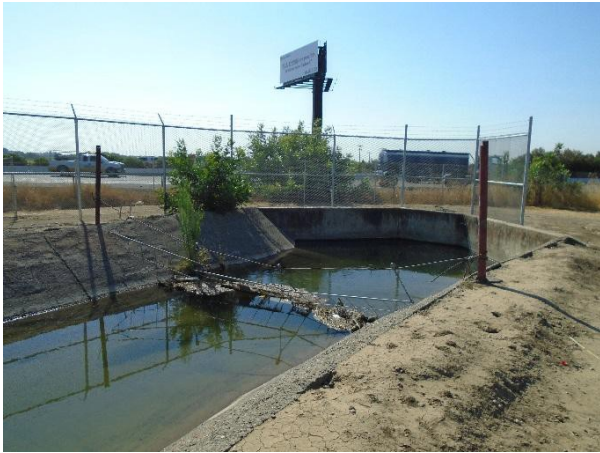
Photo 4. View of an inlet structure of the Weyand Canal at Interstate 80, facing south.
