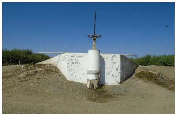
Photo 9. View of the southern terminus of the Weyand Canal and the Pipe Headworks, facing west
