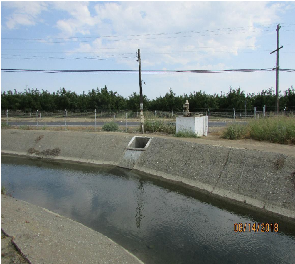
Representative Photograph 2. Inlet Structure
