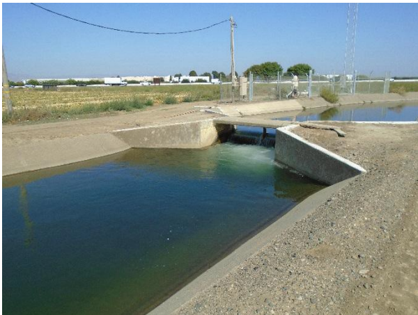
Photo 6. View of the Weyand Canal showing the Check 14 Structure and deep drainage well, facing north.
