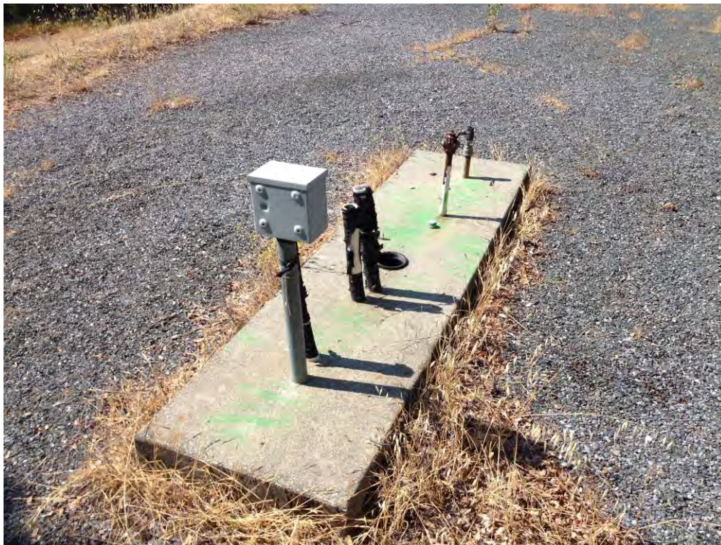
Photo 8 – Typical utility hookups in paved area upgradient of Shirland Canal
