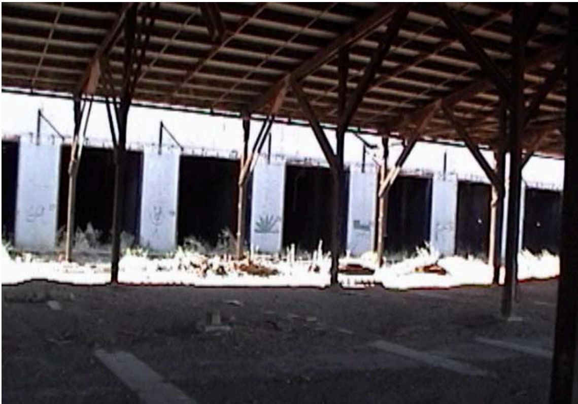
FIGURE 2 Bat Habitat—Large Bays Made of Concrete Block in Abandoned Covered Storage Building
