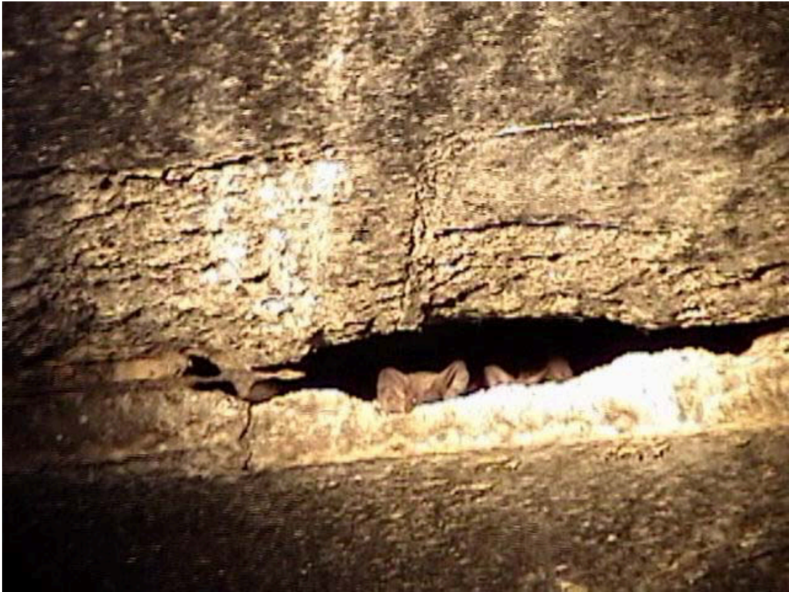
FIGURE 3 Mexican Free-tail Bats Inside Cement Wall Cavity Roost
