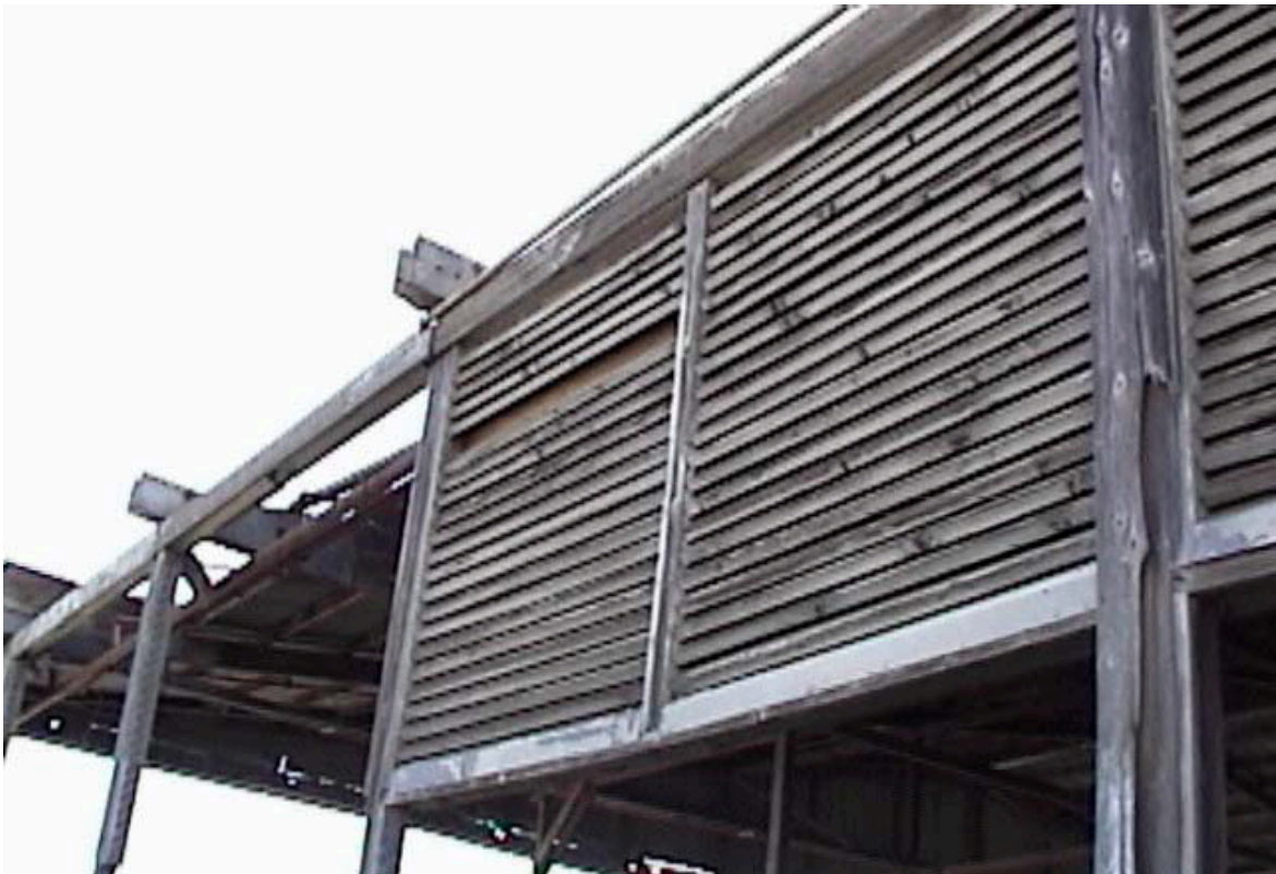
FIGURE 4 Bat Habitat—Louvered Windows Backed by Plywood and Loose Boards at Open-walled Abandoned Storage Building
