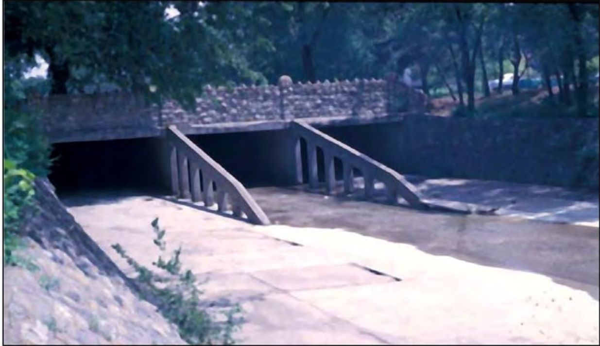
Figure 4-7. Debris Fins Incorporated at Headworks Structure (Example)
