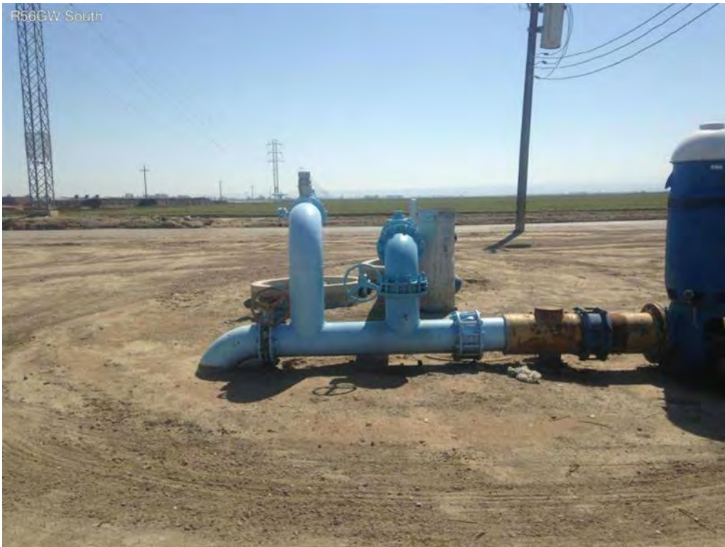
Photo 2: Representative Photo of Existing Well.
