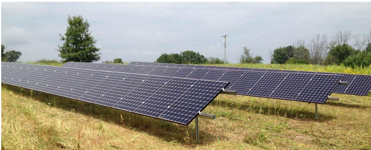
Figure 4. Typical Ground-Mounted Solar PV Panels. Source: Patriot Solar Group 2016 http://patriotsolargroup.com/solar-projects/manchester-mi-solar-installation/ .
