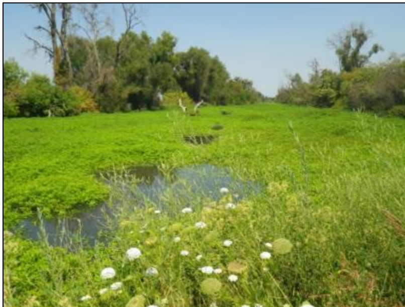
Figure 1-8 View Upstream of Agricultural Road Crossing 3, Showing Vegetation Growth Concealing an Undersized Culvert Looking North on Road Crossing
