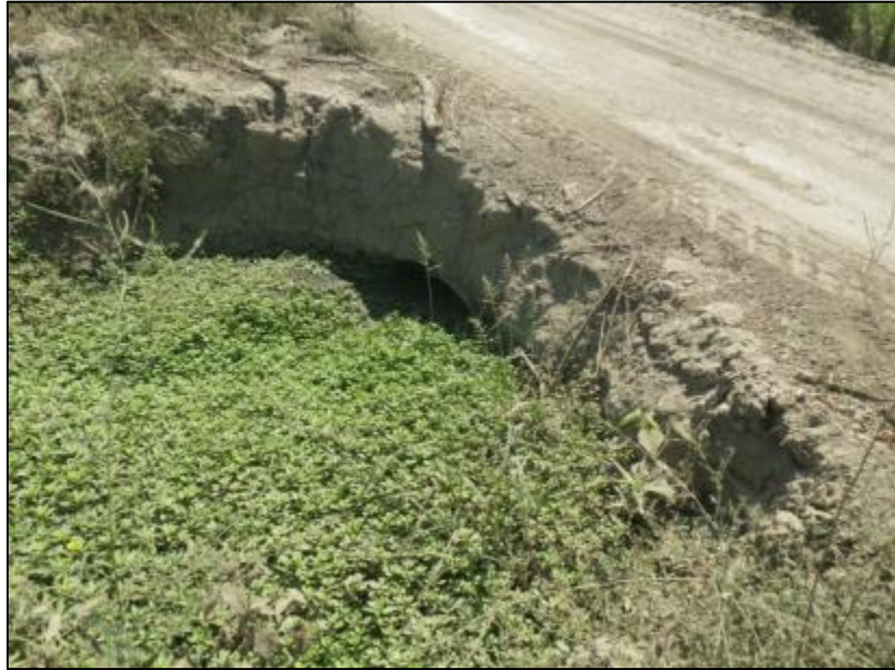
Figure 1-5 View of Upstream, Northern Face of Agricultural Road Crossing 2 (Looking South) Showing Excessive Vegetation Build-up Clogging an Undersized Culvert
