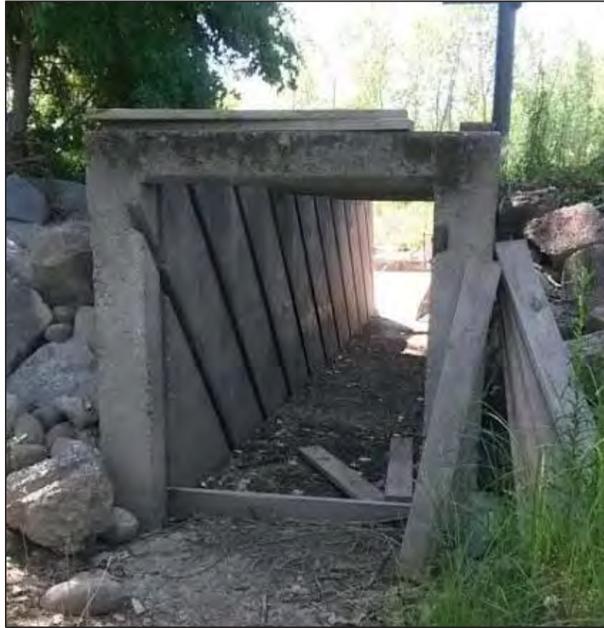
Figure 1-2 View of Existing Modified Denil-type Fish Ladder with Stoplogs and Interior Baffles Removed, Looking Downstream
