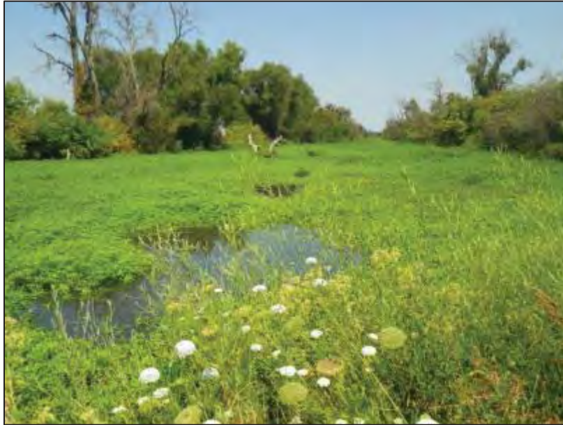
Figure 1-8 View Upstream of Agricultural Road Crossing 3, Showing Vegetation Growth Concealing an Undersized Culvert Looking North on Road Crossing
