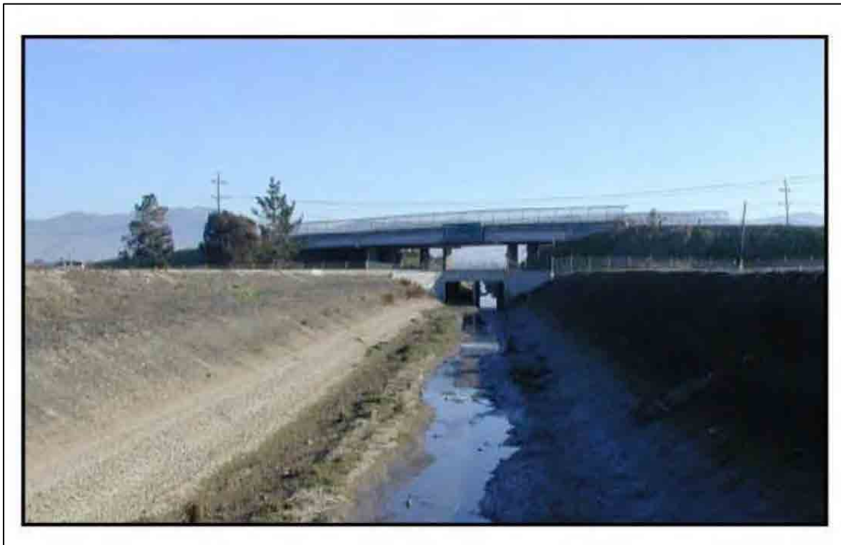
Figure 6-2. Typical ditch-like channel conditions in Action Area of Reclamation Ditch.
