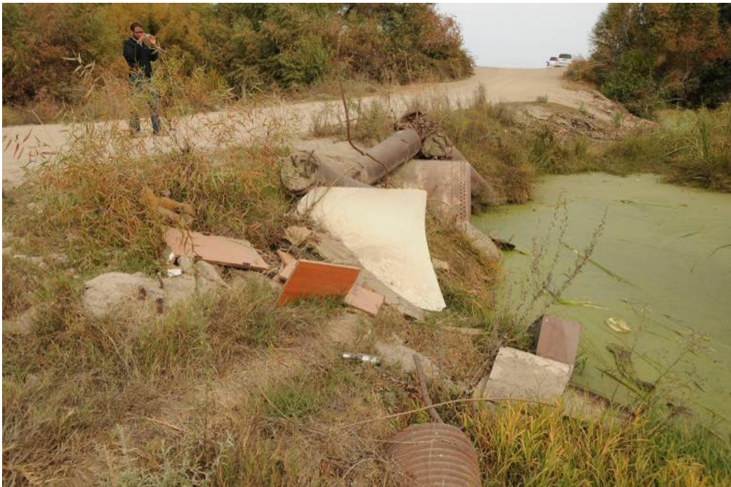
Figure 1-8. San Mateo Avenue crossing of Reach 2B showing single culvert beneath the road (12/15/09)
