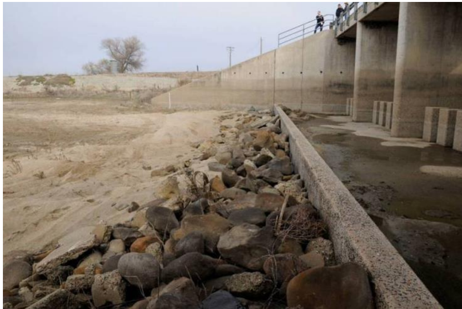
Figure 1-6. Concrete sill and bordering riprap along the downstream edge of the Chowchilla Bifurcation Structure in Reach 2B 3 (12/15/09)
